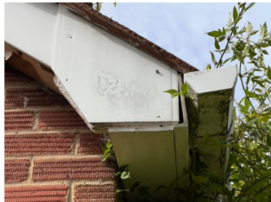
33: Gap in the fascia board.
