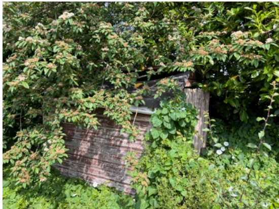
40: Dilapidated shed towards the north of the site.
