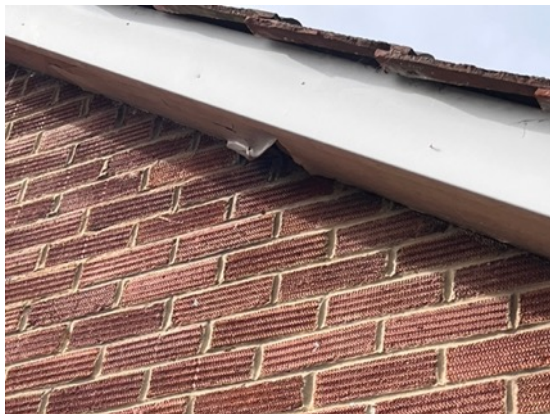
32: Damaged barge board.
