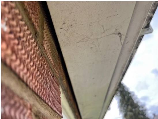
36: Gaps between the wall and soffit box on the west elevation.
