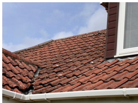
35: Gaps under tiles on south elevation.
