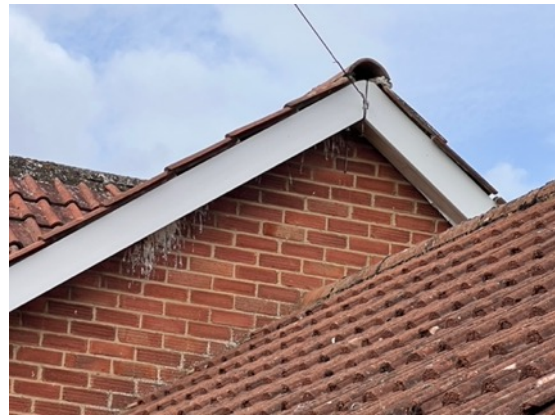
37: Gaps under tiles on the verges on the east facing gable end.
