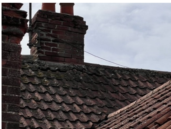
34: Gaps under tiles on the north elevation.
