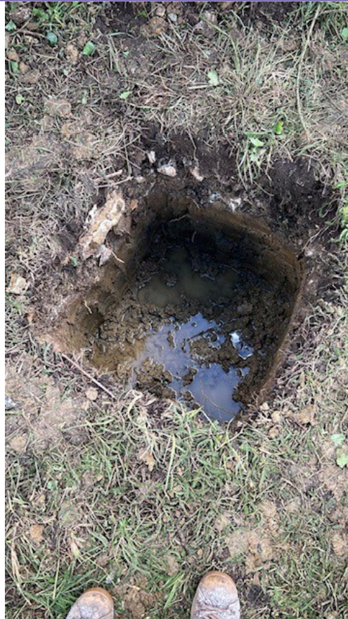
Photograph 1: Showing clay strata beneath topsoil and accumulated water
