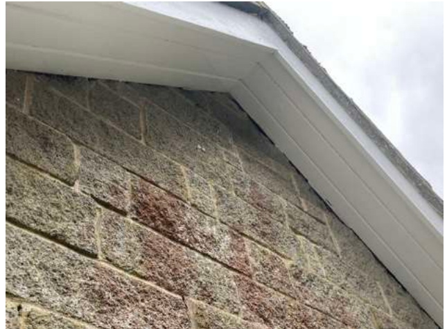
Image 2: Gaps in the soffit box which were subjected to a high level inspection.
