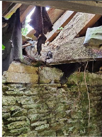
Failed truss bearing
