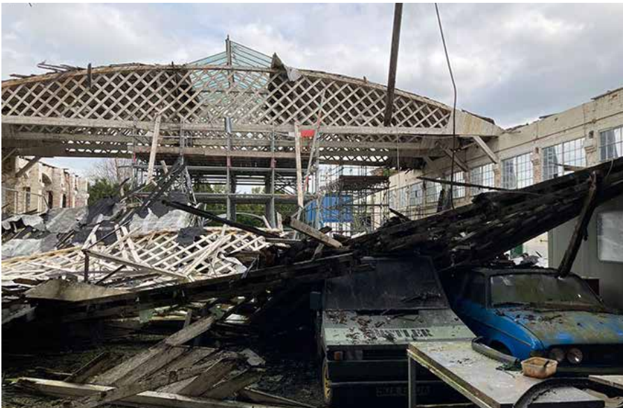
Area of collapsed roof
