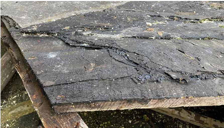
Existing roof build-up from collapsed section
