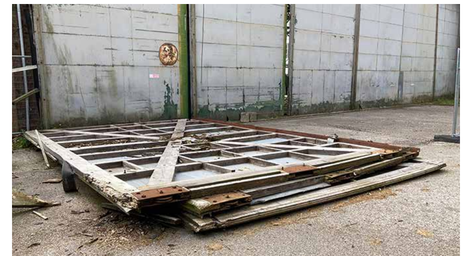
Collapsed hangar doors.
