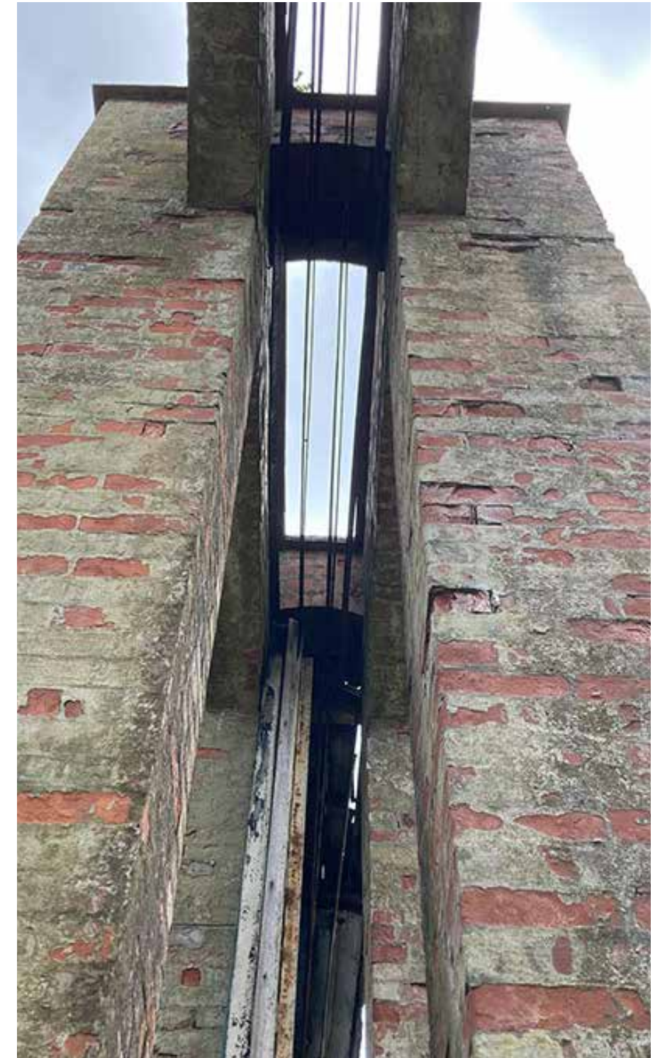
Gantry tower showing door running gear
