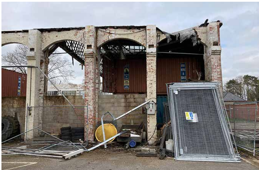
Central brick arcading with missing roof
