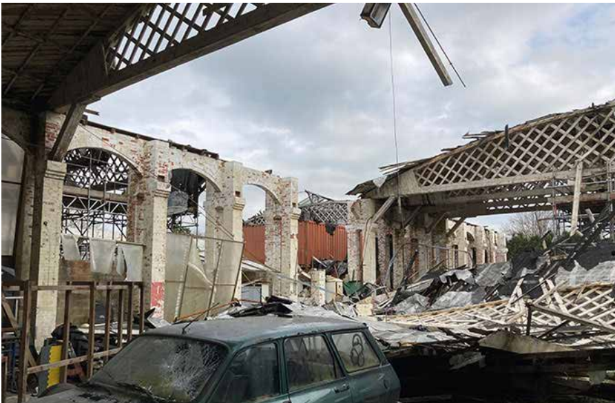
Area of collapsed roof
