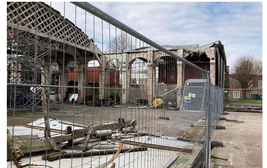
Worst area of collapse
