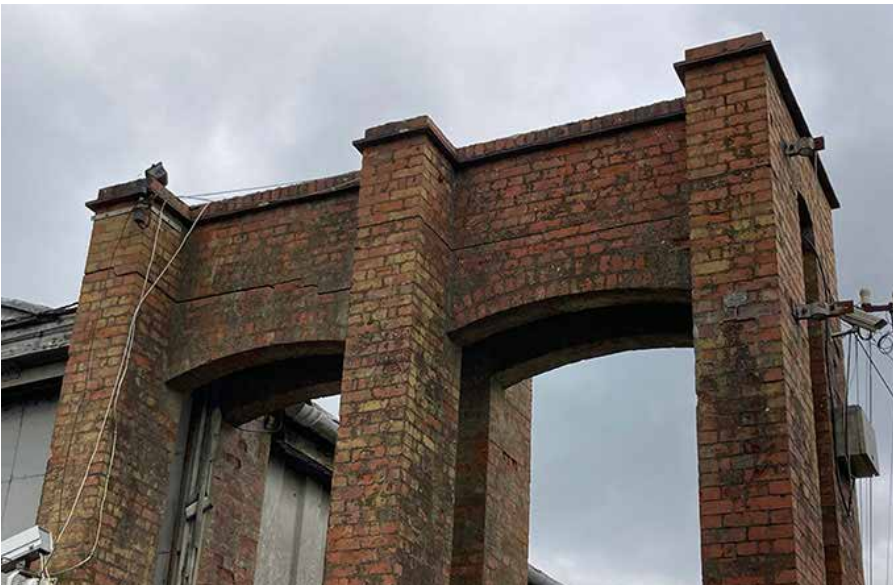
Top of gantry tower showing horizontal cracking
