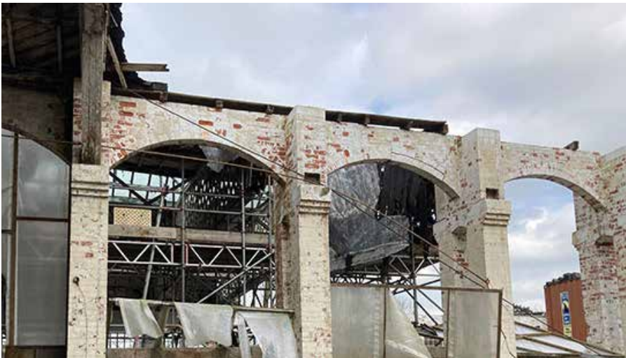
Central brick arcading in need of brick repairs
