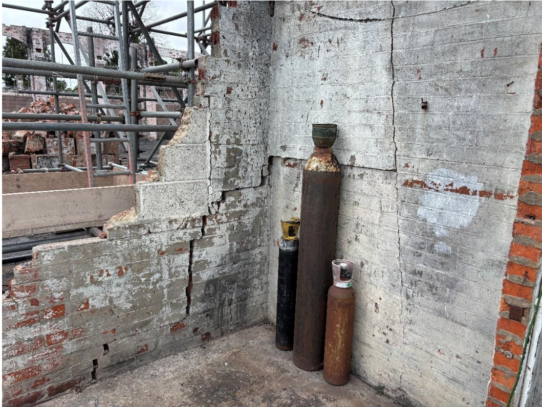
Figure 28 Cracking to buttress on GL16
