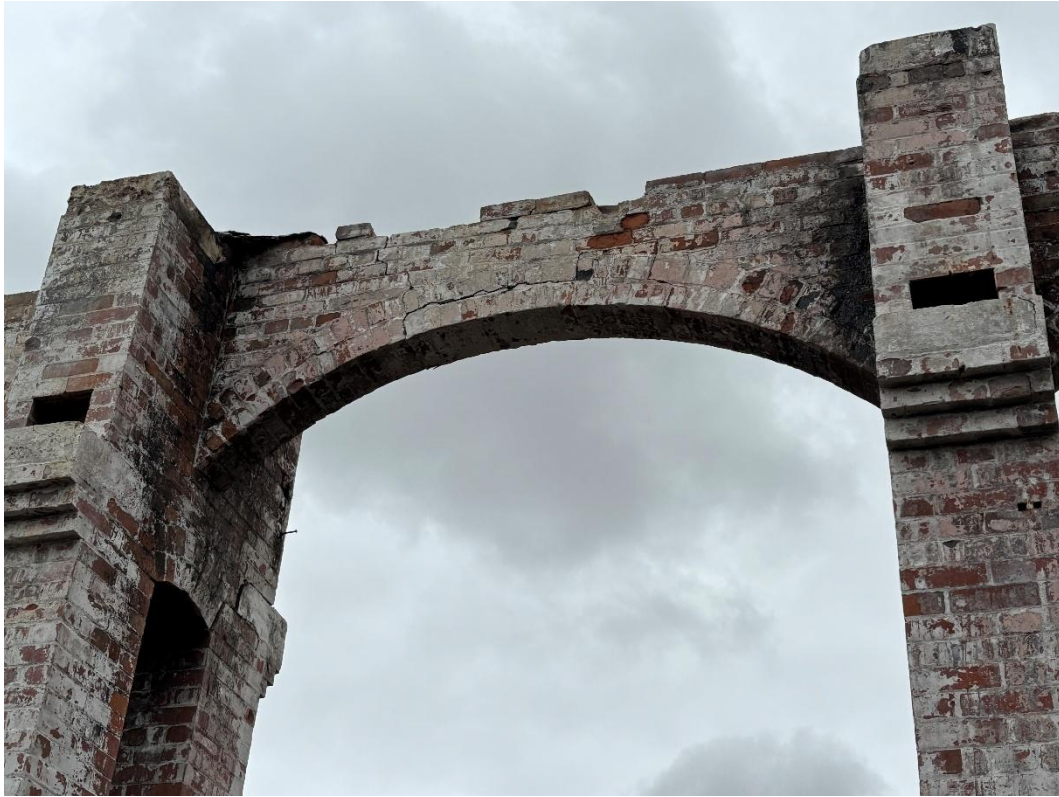
Figure 35 Cracking the arch between GL15 and GL16
