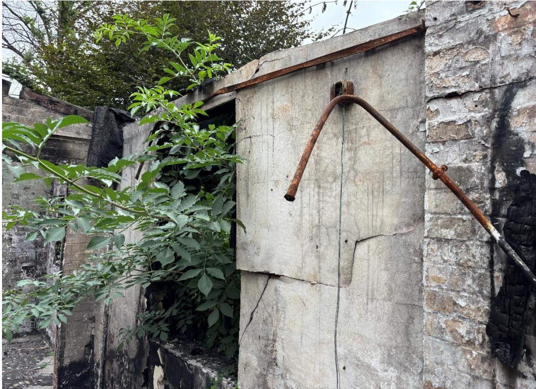
Figure 38 Example of inner blockwork and brick skin separating
