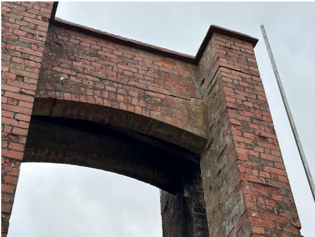
Figure 15 Cracking to the top of door support piers and connecting arches
