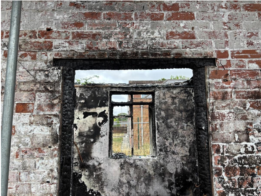
Figure 16 Example of fire damaged timber lintel
