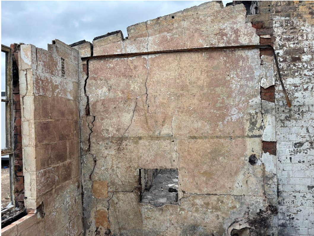
Figure 45 Cracking between cross wall and external wall showing external wall leaning to left
