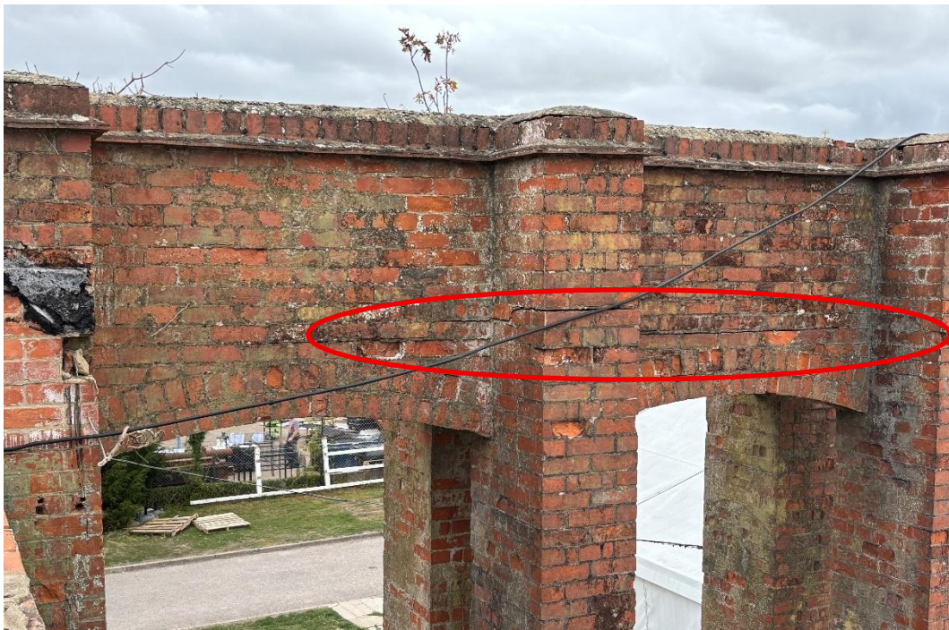
Figure 20 Cracking to northern door support piers
