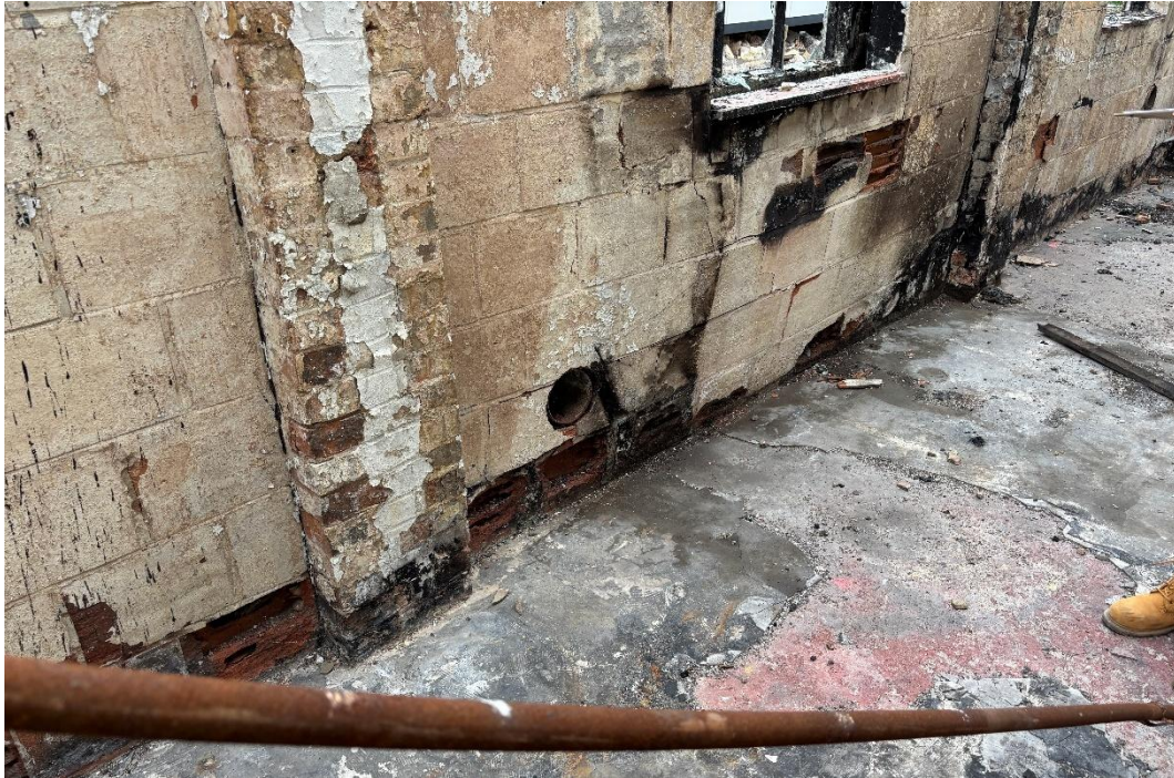
Figure 43 Example of inner clay block separating from brick outer leaf
