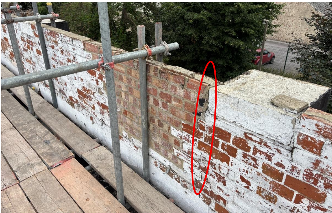
Figure 7 Example of past brick repair and vertical crack between buttress and wall panel
