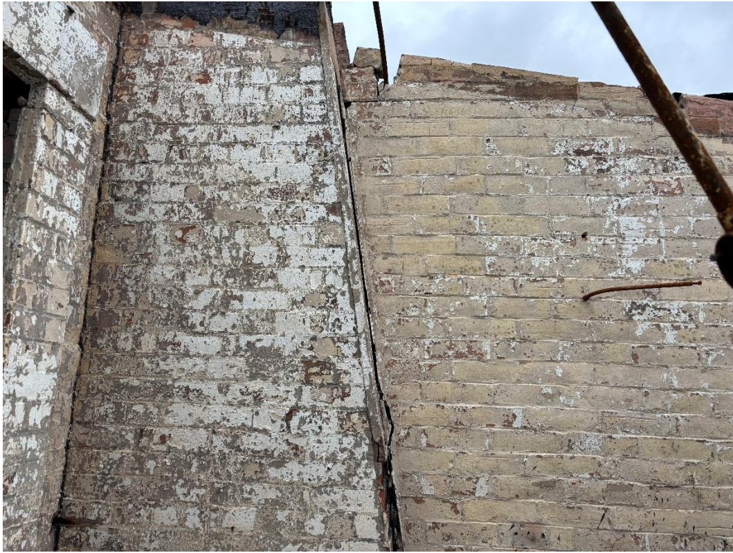
Figure 40 Dividing wall separating from buttress
