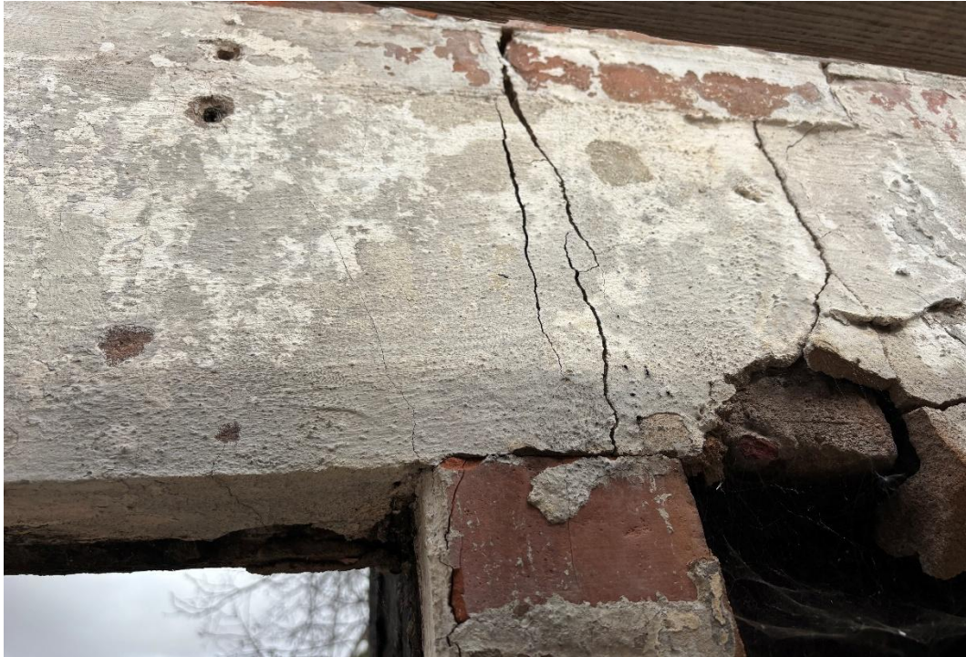
Figure 8 Lintel crack GL11
