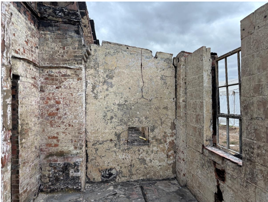
Figure 44 Cracking to masonry cross wall
