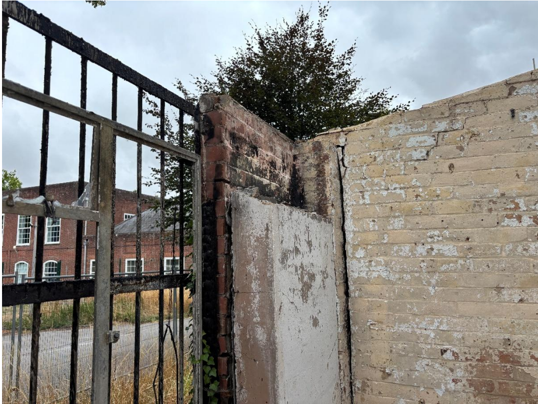
Figure 41 Cracking between dividing wall and external wall showing external wall leaning to left
