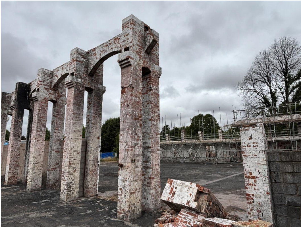
Figure 34 Collapsed pier GL09
