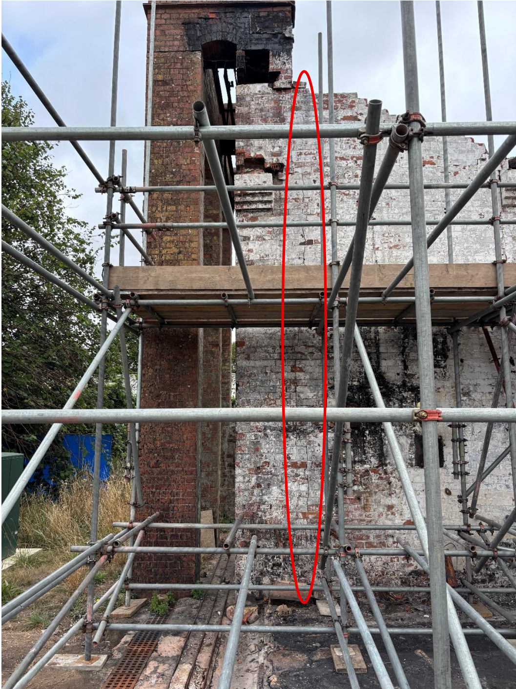
Figure 13 Crack between wall panel and door support piers on GL17
