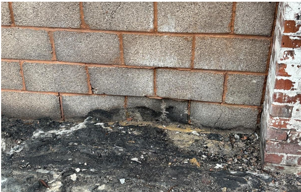
Figure 33 Damage to blockwork panel GL05 to GL06
