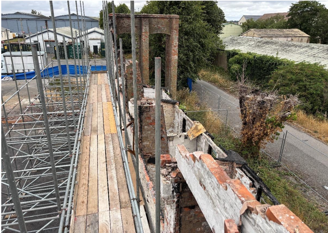
Figure 10 Masonry collapse between GL11 and GL17
