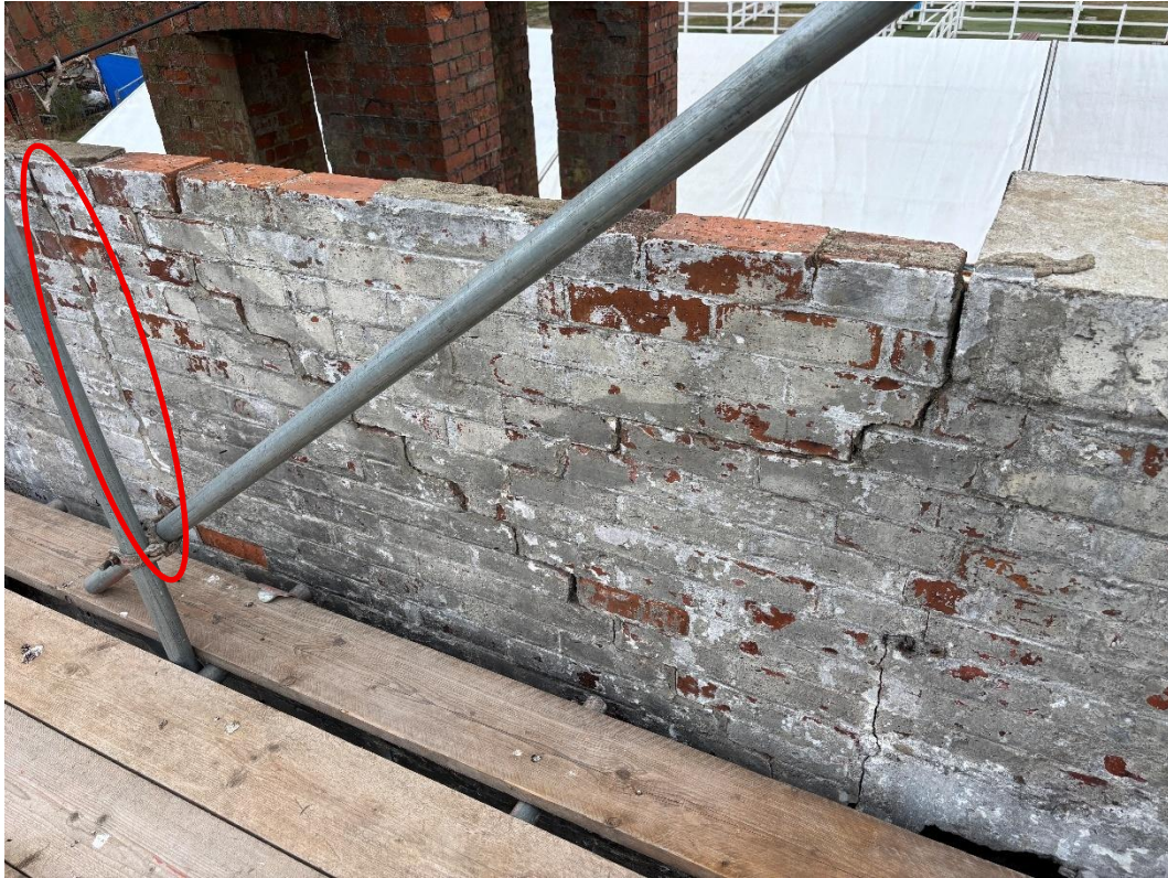
Figure 22 High level cracking between GL01 and GL02 including historic repaired cracks
