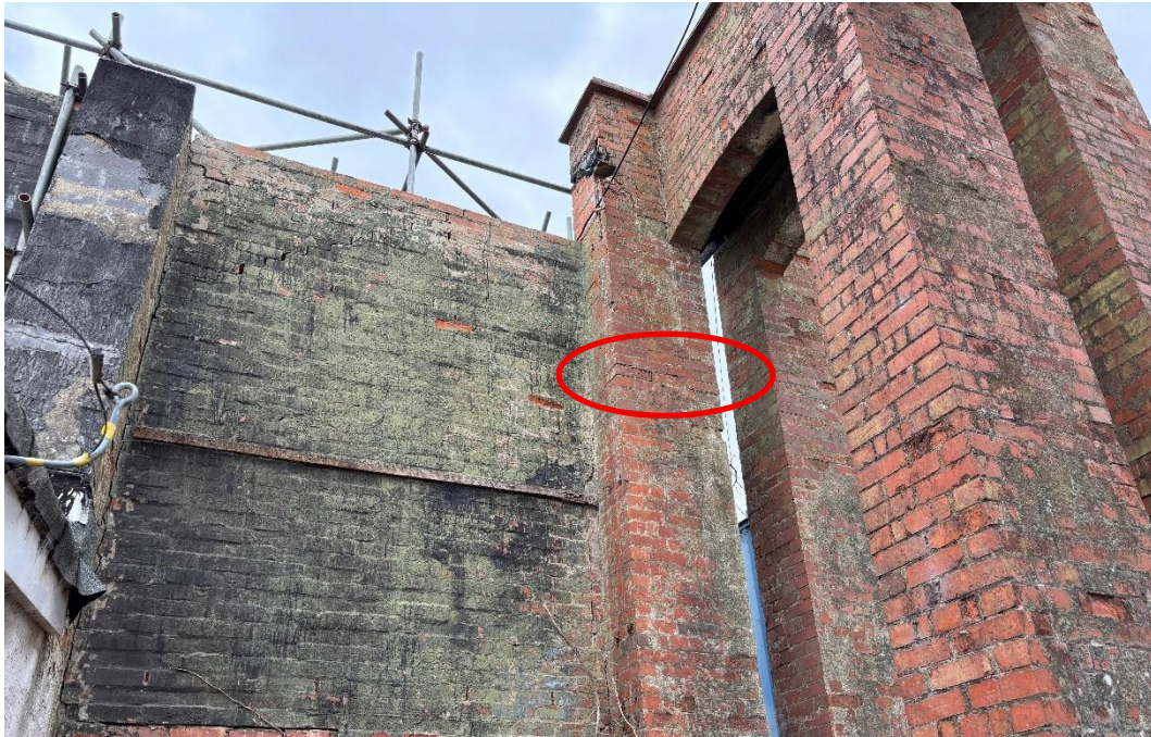
Figure 19 Cracking to northern door support piers
