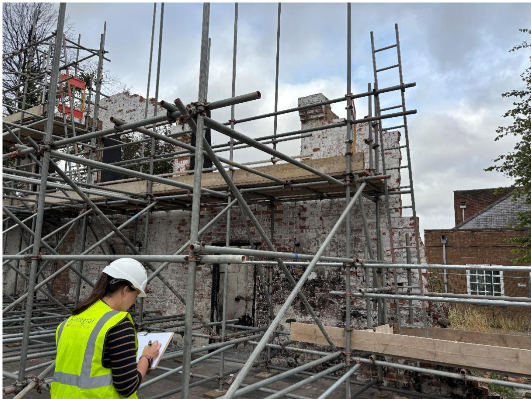
Figure 5 Wall collapse between GL01 and GL03
