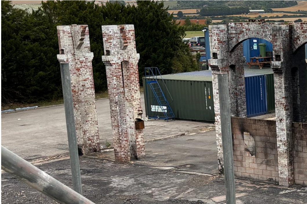
Figure 32 Collapsed pier and arches GL01 to GL04
