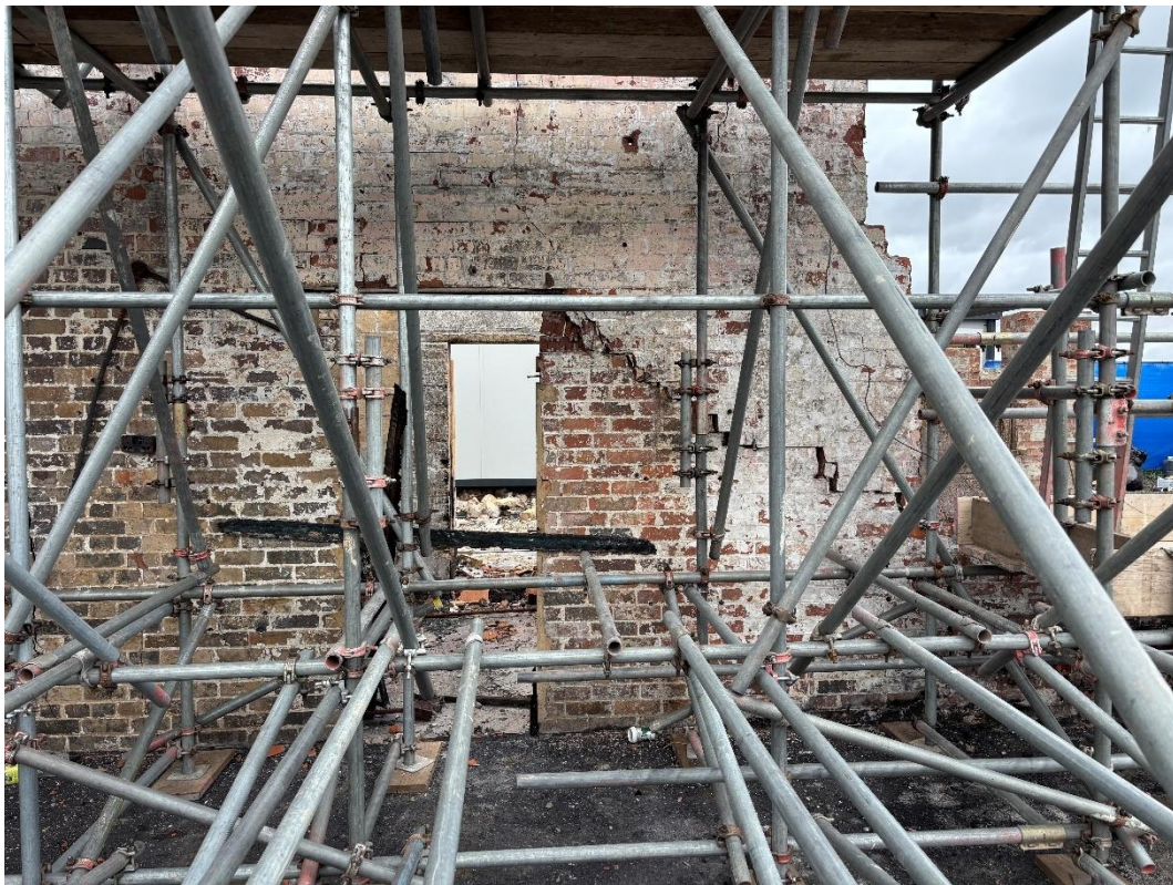
Figure 27 Cracking to southern end of wall (GL15 – GL17). Collapsed section of wall to right hand side of image
