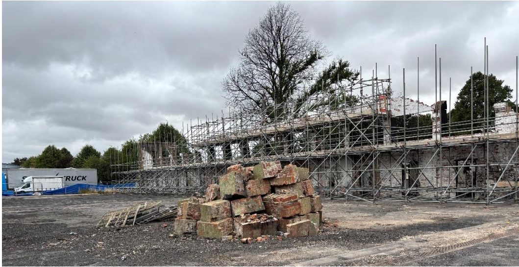
Figure 6 Masonry stored on site from collapsed door support piers
