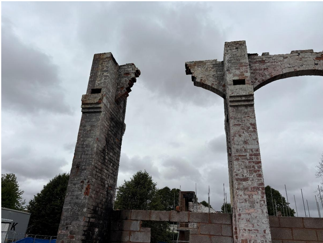
Figure 36 Collapsed arch GL16 to GL17
