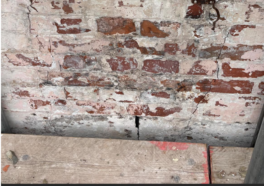
Figure 25 Cracking to lintel bearings GL11
