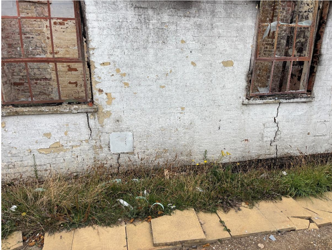
Figure 46 Example of cracking the external wall
