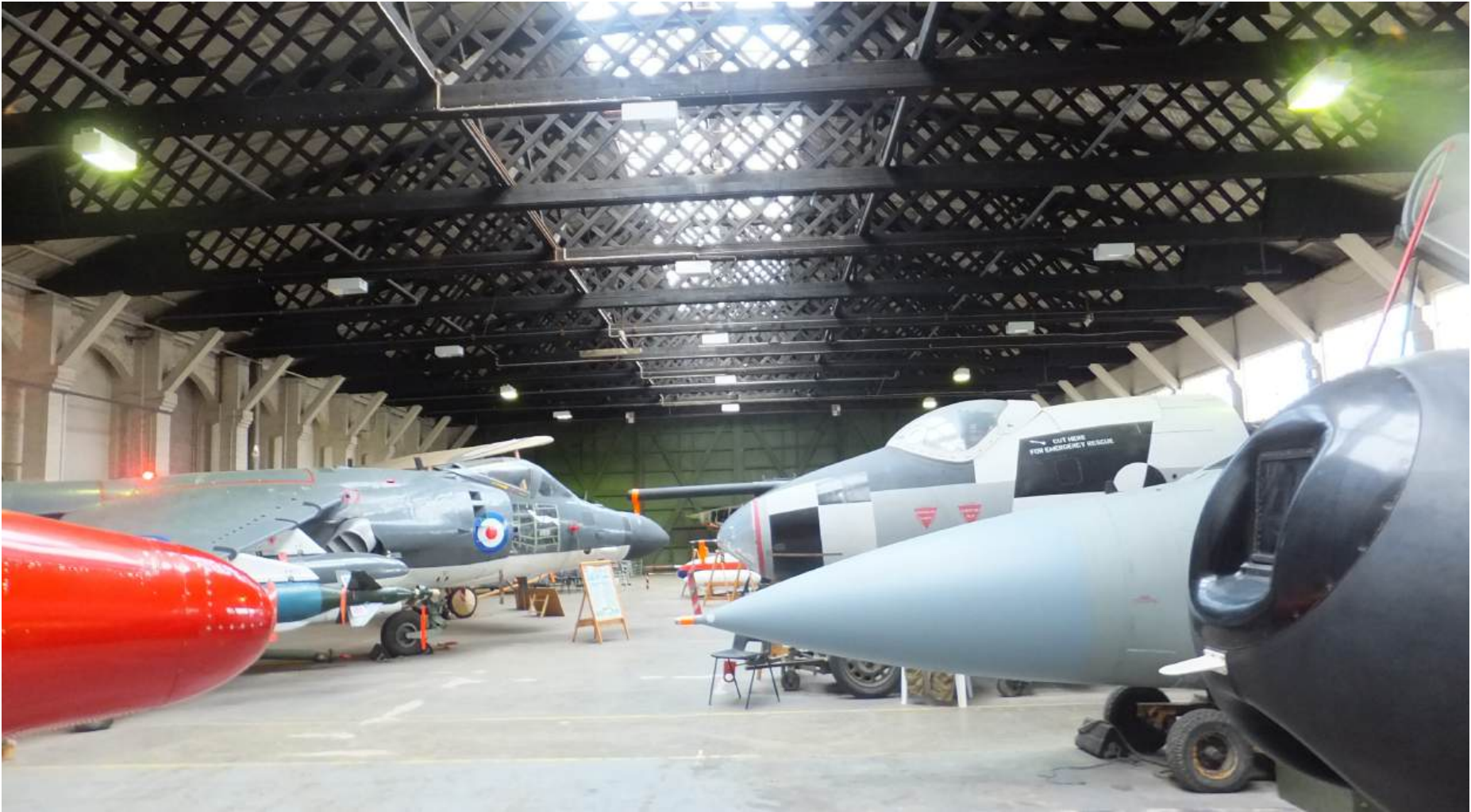
Interior of the south bay Belfast trusses treated with creosote during late 20th century
