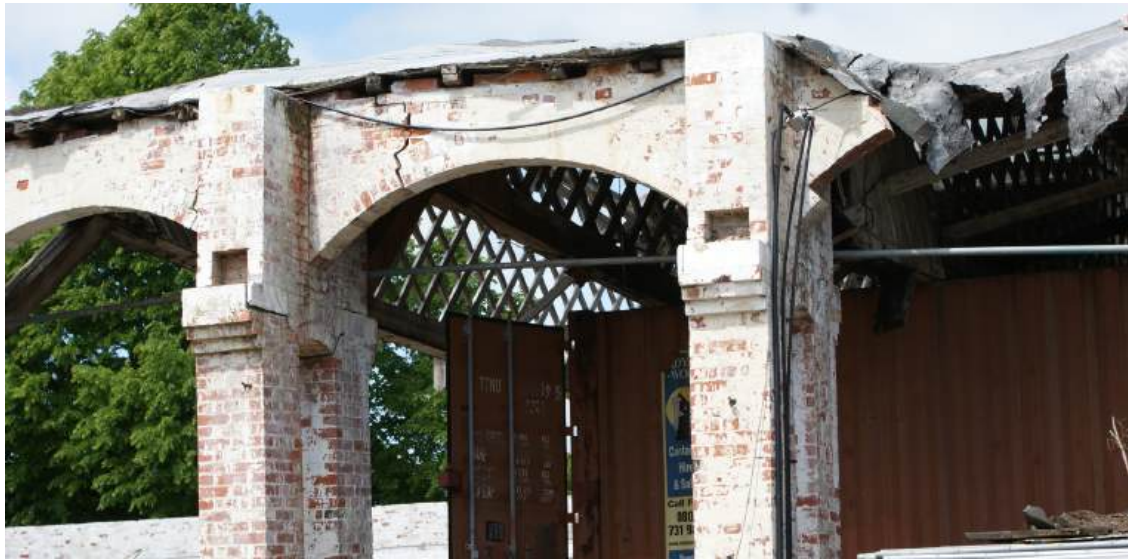
Dividing wall and collapsed roof truss
