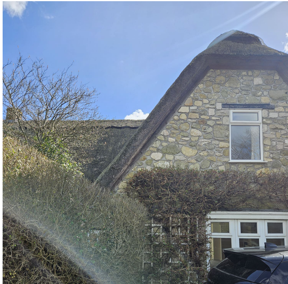
Fig 5. NW gable with poor quality stonework. This gable replaced a former brick gable, see next image.
