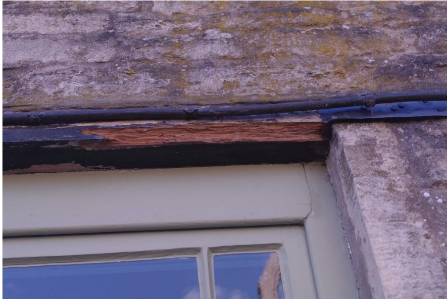
Figure 4: View of the rotten timber lintel at the front.
