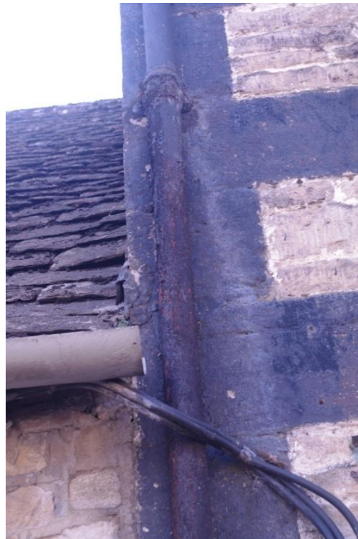
Figure 3: Heavily corroded downpipe to be replaced like for like.
