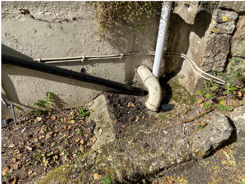
Property drainage mid slope on northern boundary
