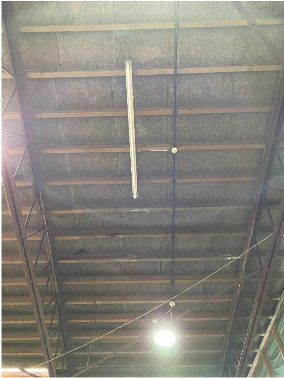
Roof within extension to garage – possible ACM
