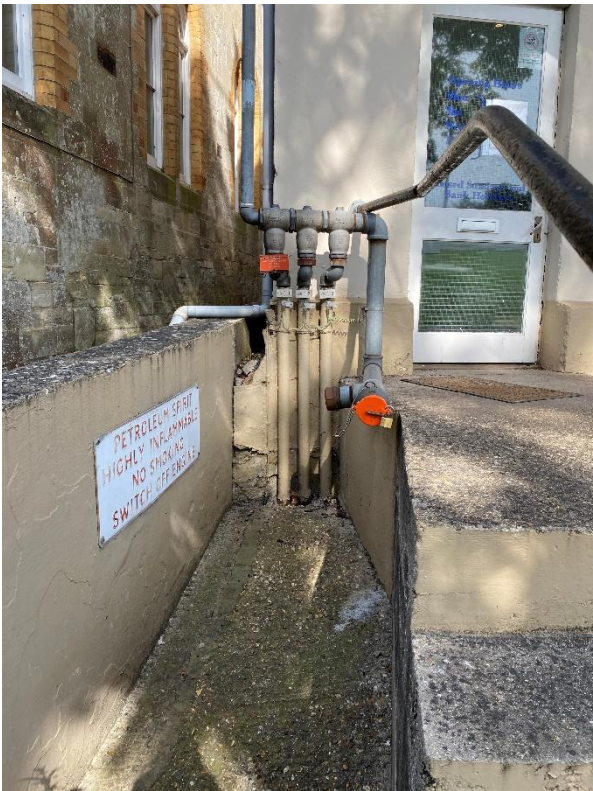
Fuel filling points at southern boundary
