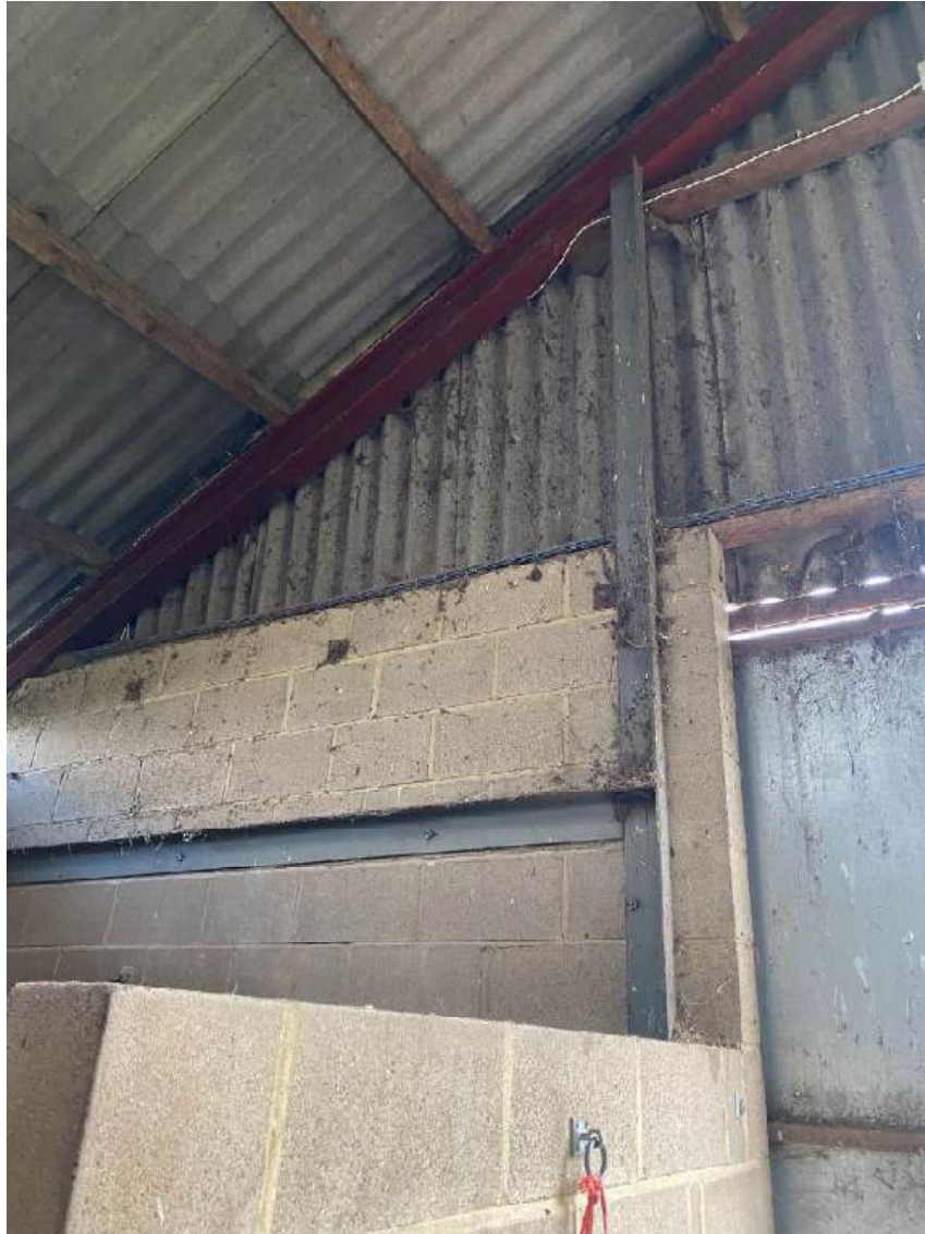
Figure 1.13 – Steel frame bolted to wall supporting sliding doors
