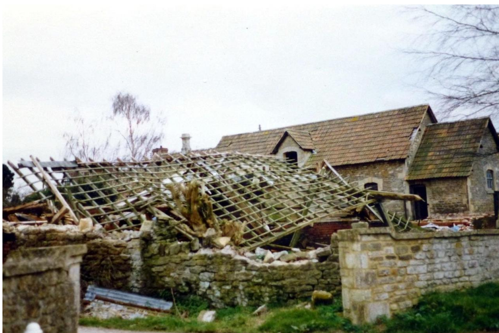
Figure 7 - This shows the collapse of the listed barn facing Main Street, which occurred in the storm of October 1987. The Old Stables is in the background.
