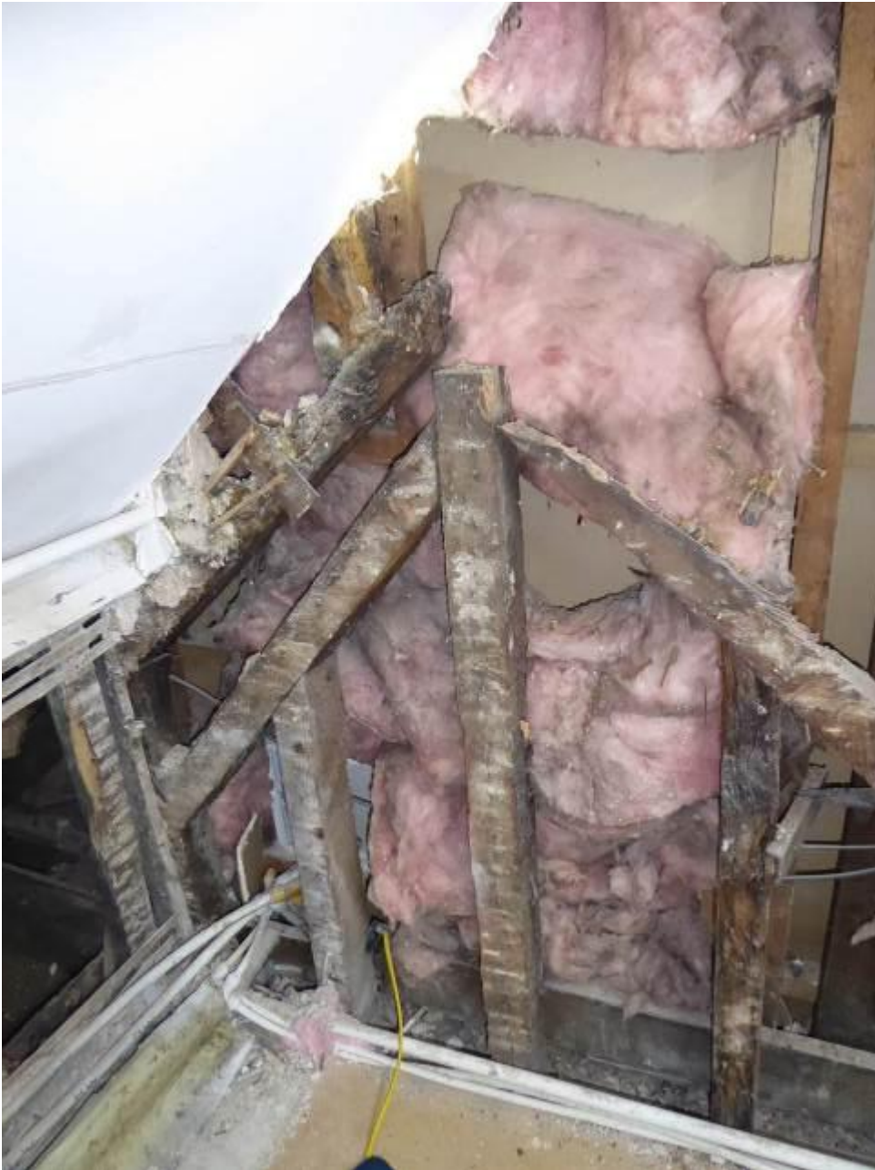
Failed roof support framing above bar beam
