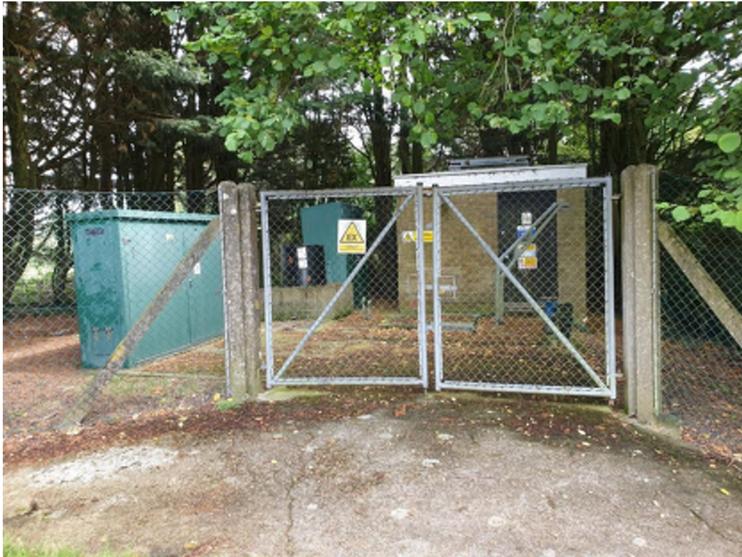
Southern Water Foul Pumping Station
