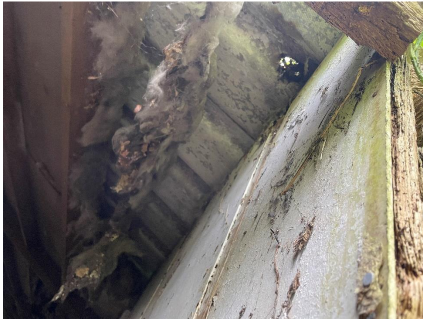
Photograph 8: Hole in the roofing sheet of B1
