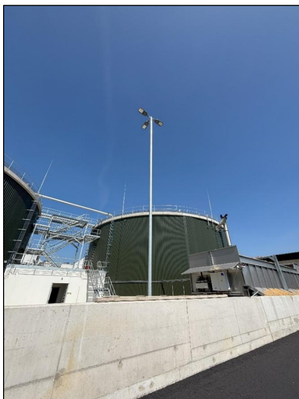
Figure 17: HVI Conductors to Flat Roof Digesters
