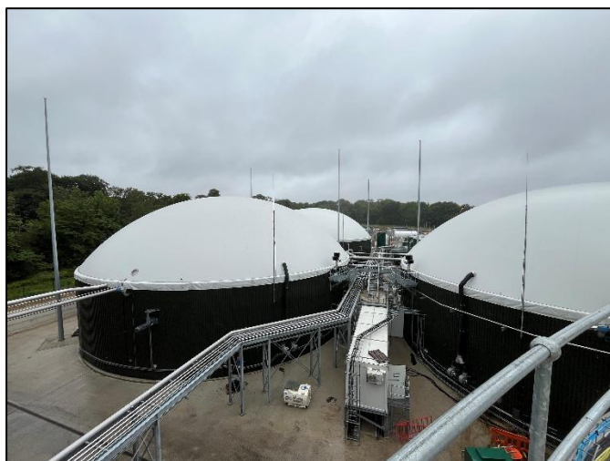
Figure 15: HVI Conductors and a Telescopic Mast to Digesters
