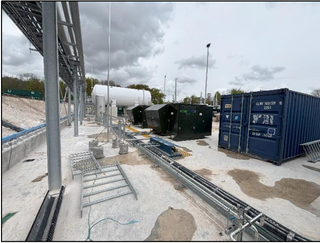
Figure 19: Self-Supported Mast in Gas Area
