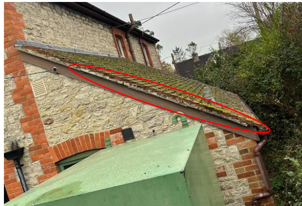
Photo 2: lower roof void to be removed.
