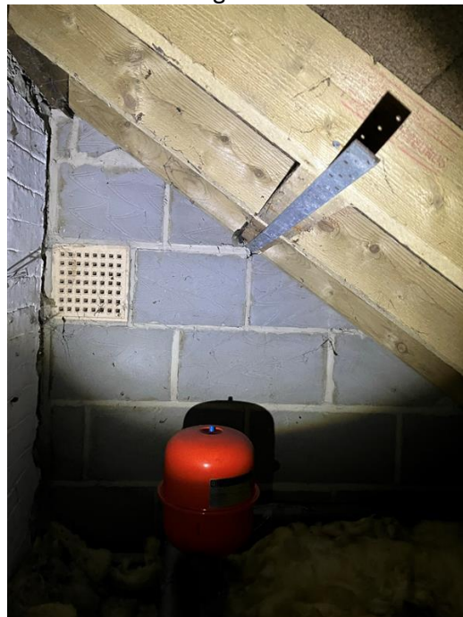
Photo 6: visible degradation around gable ends of downstairs roof void.
