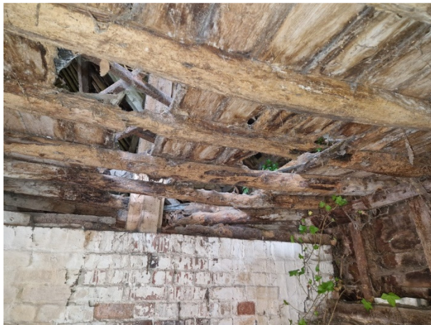
Decay in joists at northern end of main barn
