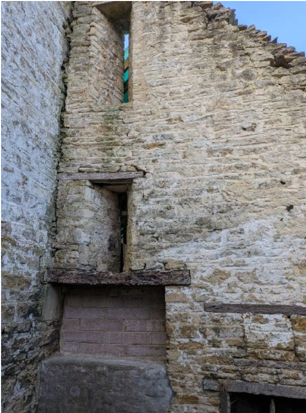
22. The Lean-to showing vertical cracks
