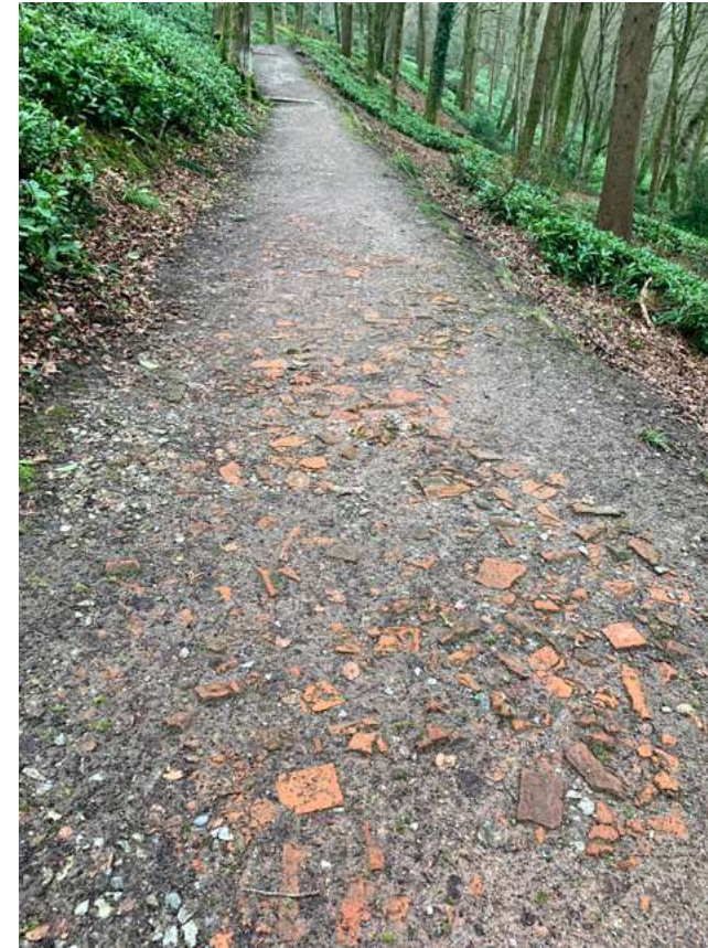
Path within the shades showing historic used of brick as a material for repair, which is being eroded away.
