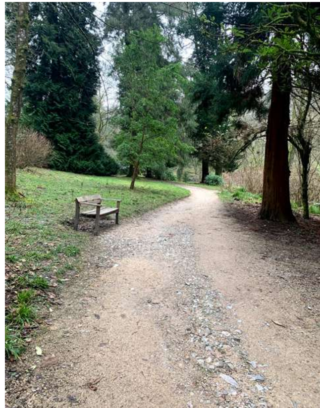
Path above the grotto with rubble substrate visible following erosion of top layers of gravel.
