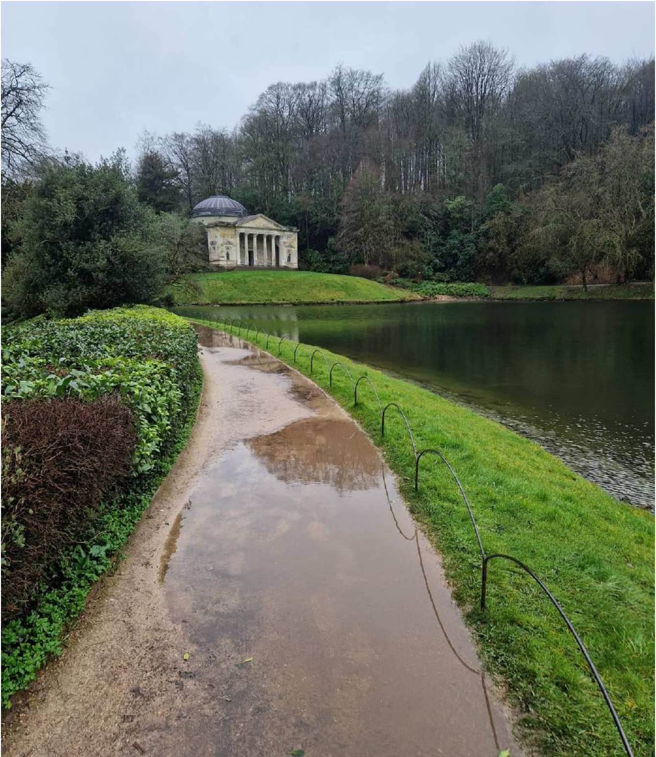
Pooling on the Dam looking towards the Pantheon
