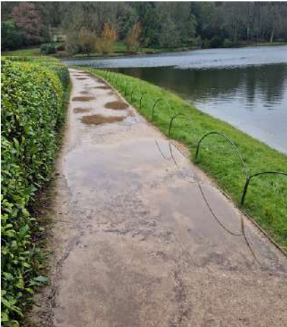
Ponding along the dam
