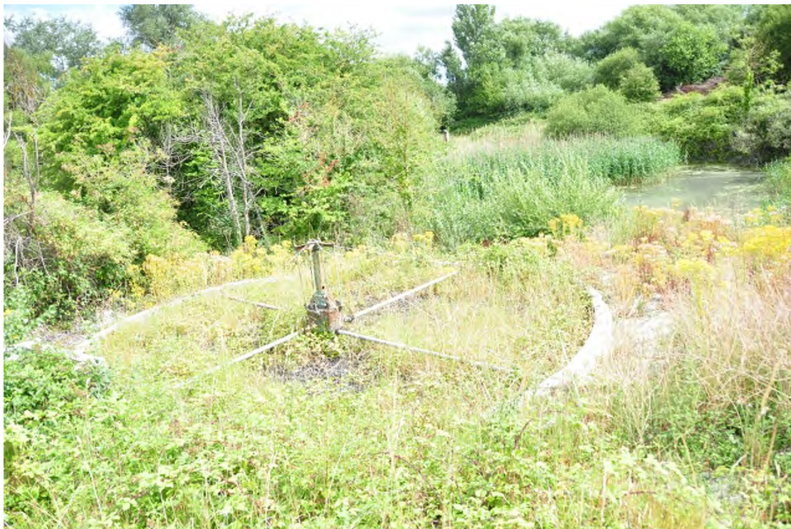
Plate 8 STW overgrown with vegetation
