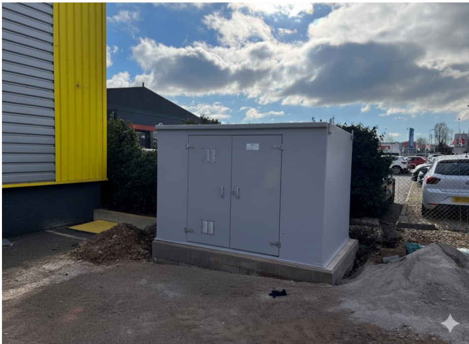
Image of typical GRP electrical enclosure
