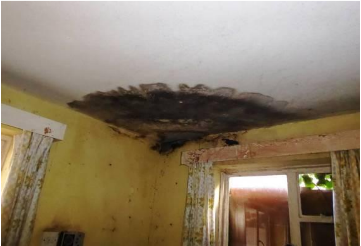
Fig 4.11.3: dry rot to ceiling and walls
