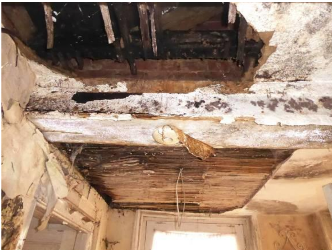
Fig 4.8.8: Collapsed ceiling and failed service block roof junction to main house
