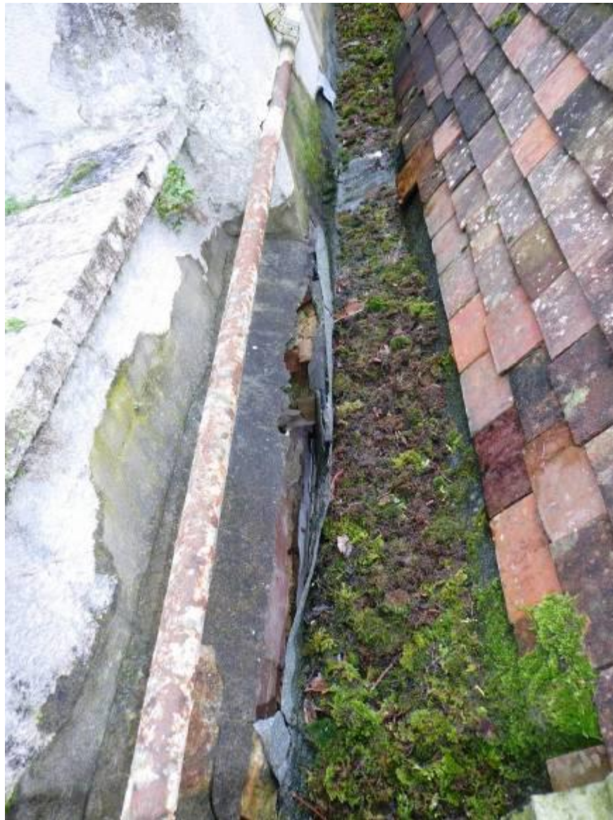
Fig 3.4.8: Failed valley gutter to north side of service block
