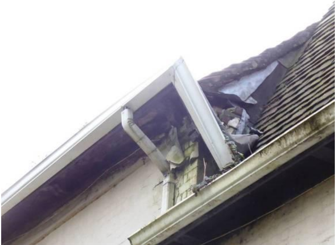
Fig 3.4.4: Collapsed gable wall head and eaves
