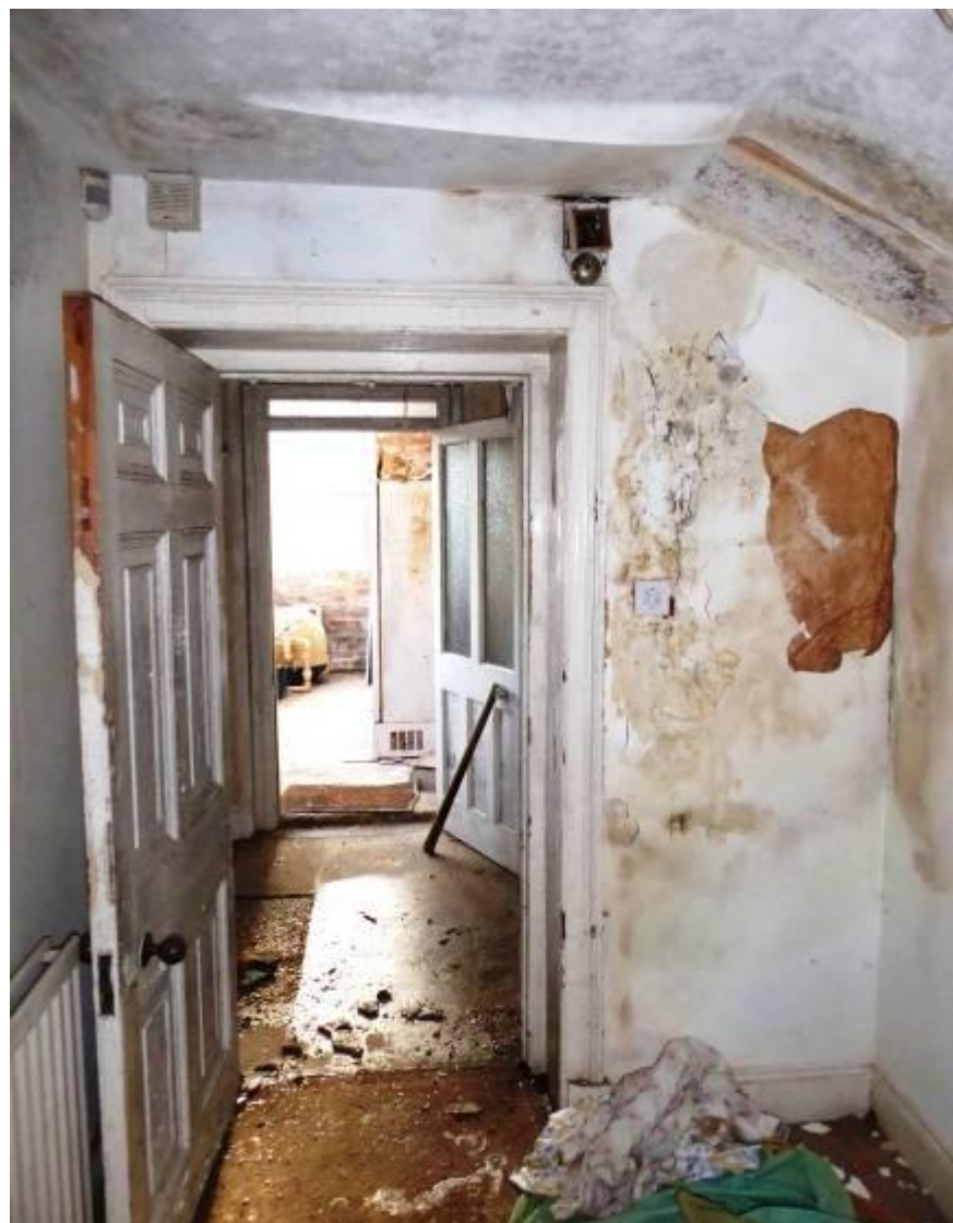
Fig 4.1.6: Severe damp entry and dry root to rear of entrance hall
