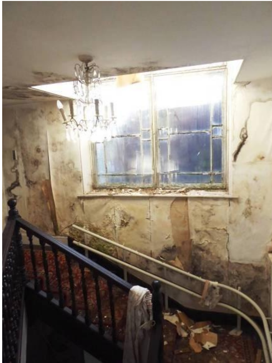
Fig 4.14.4: Severe damp damage to wall and ceiling over stairs
