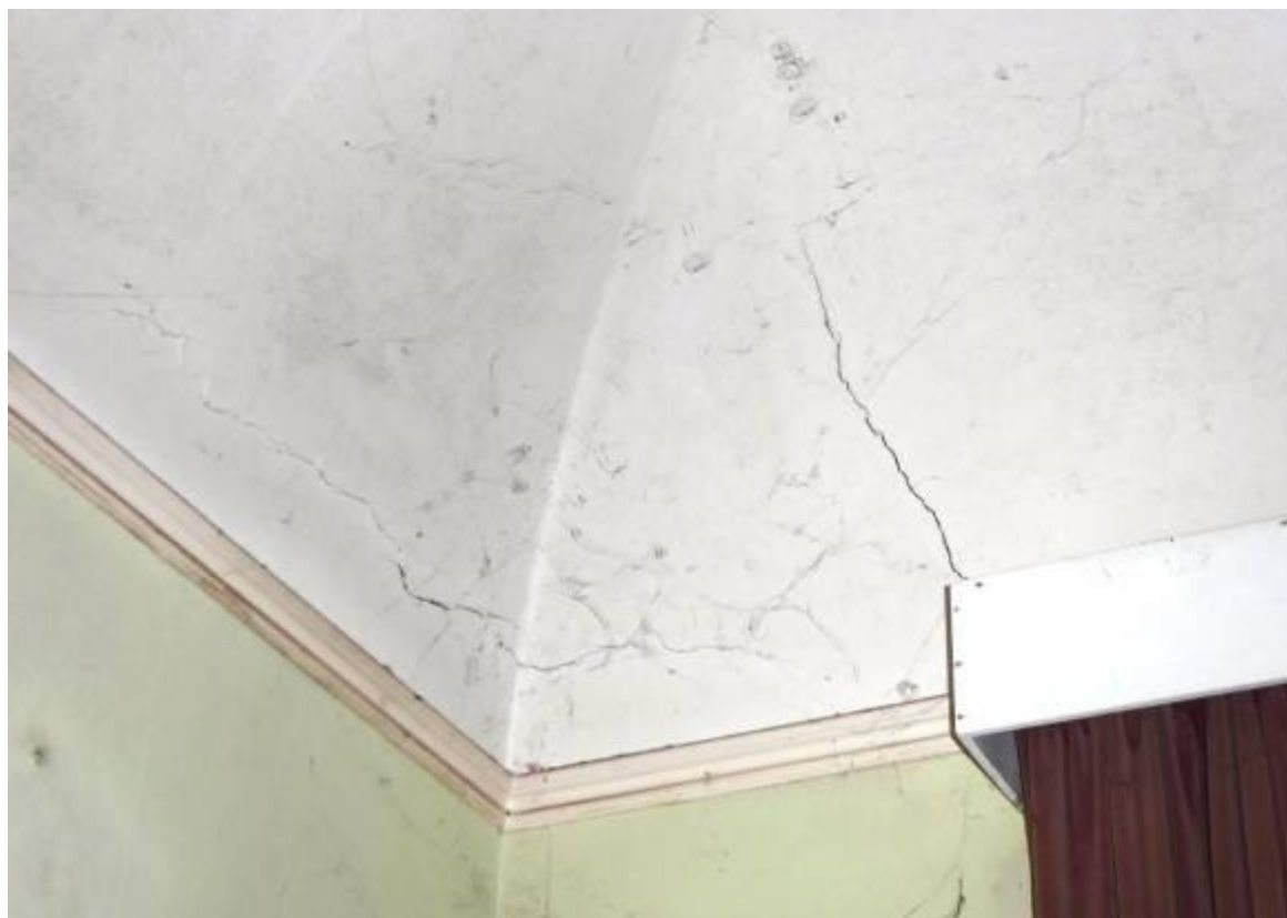
Fig 4.3.6: High level cracking and movement
