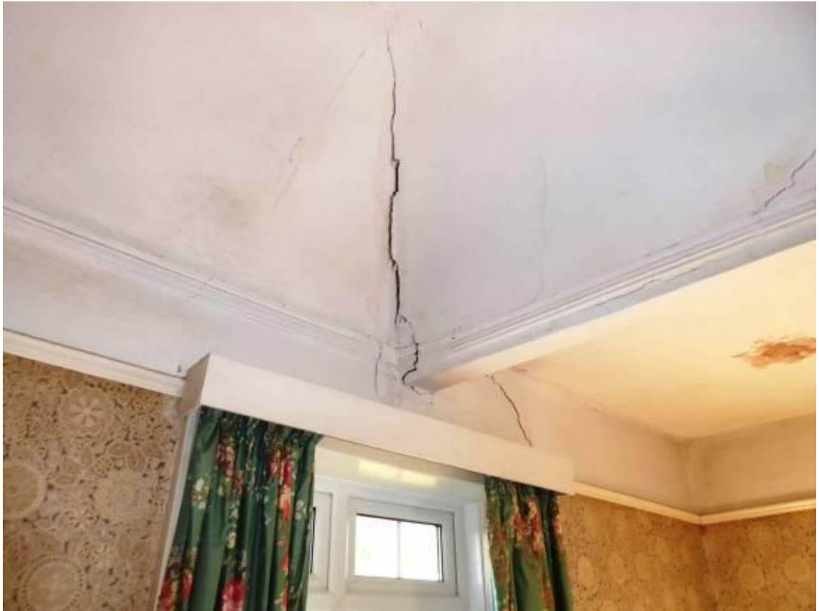
Fig 4.21.7: Severe cracking to beam end and walls
