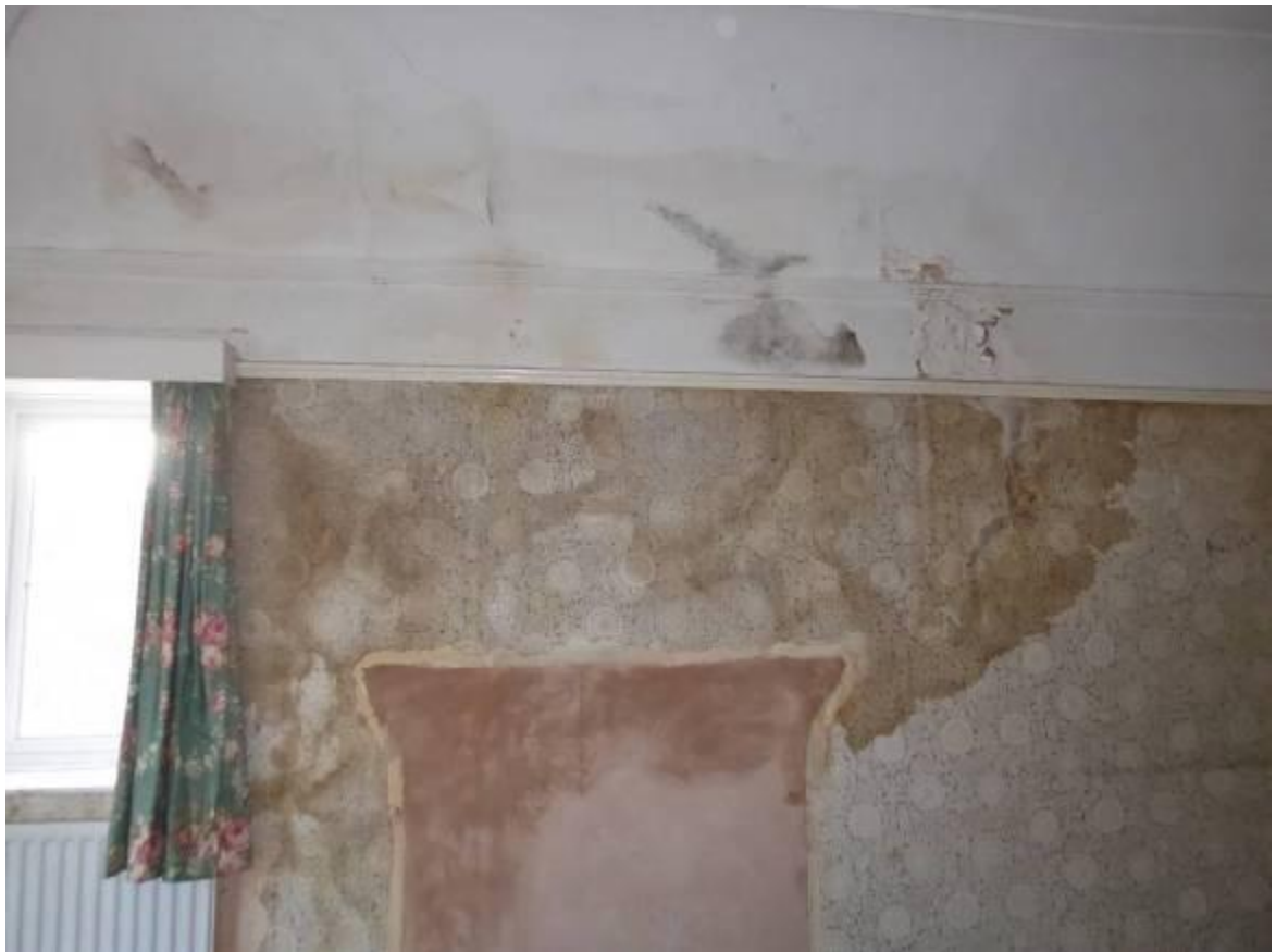
Fig 4.21.12: Damp entry to ceiling and walls
