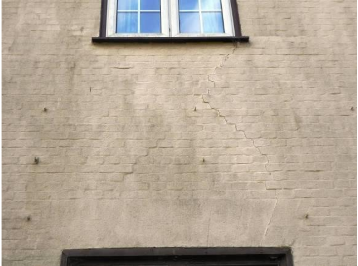
Fig 3.5.9: Cracking in north wall of east two storey part
