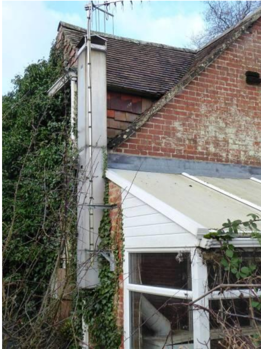
Fig 3.3.5: Swimming pool boiler flue
