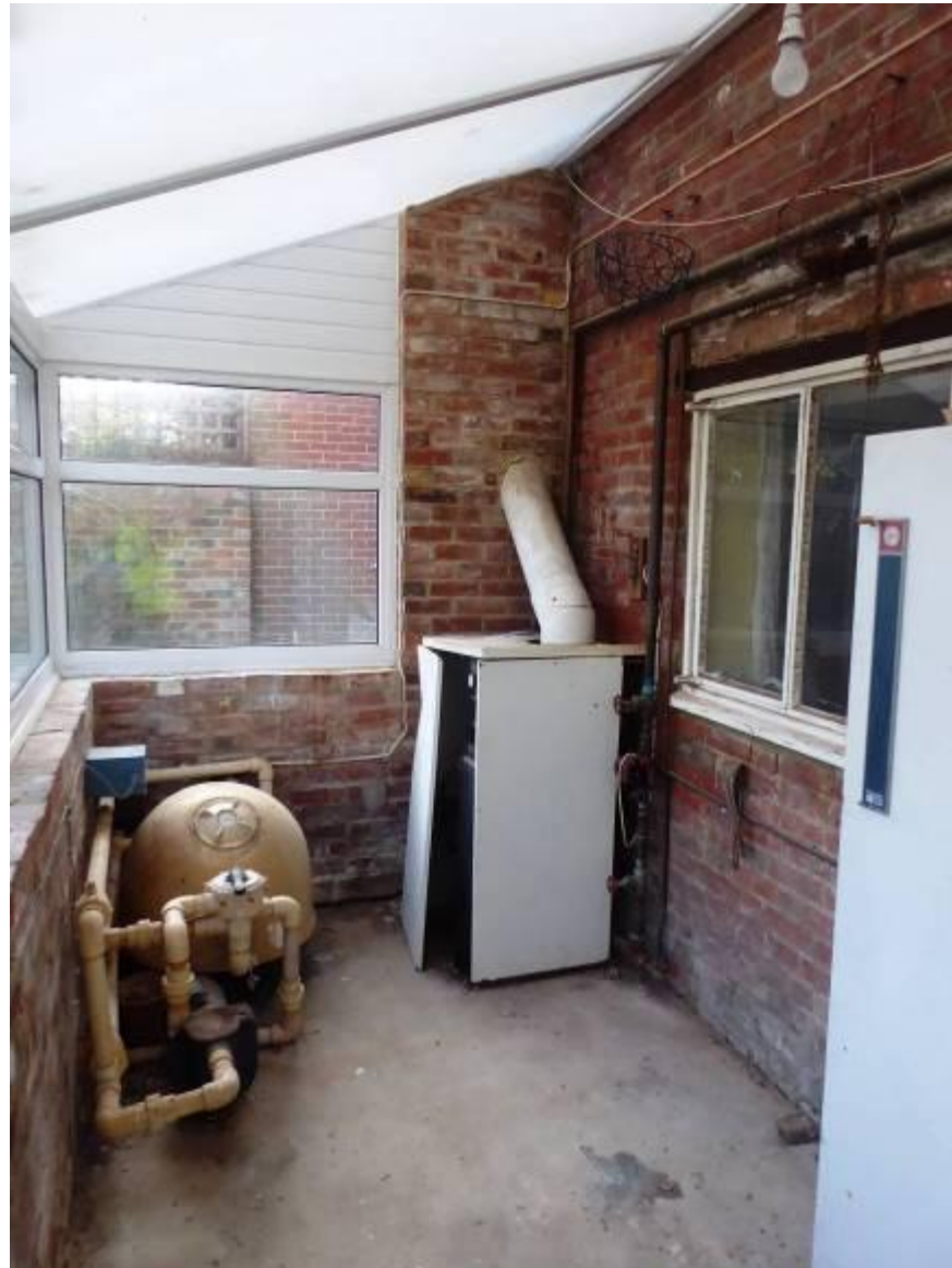
Fig 4.10: Swimming pool plant room
