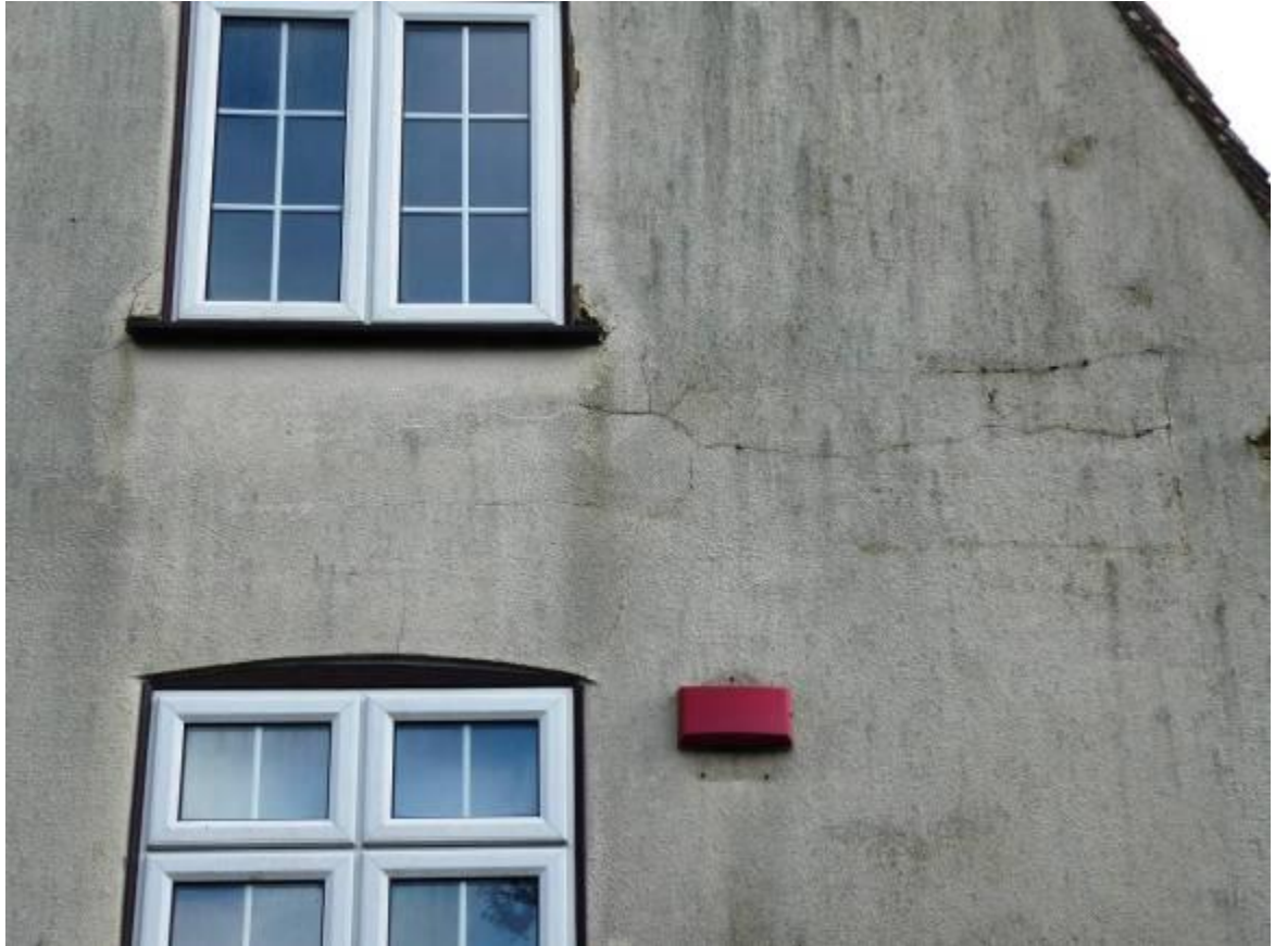
Fig 3.5.2: Cracking and movement in west wall
