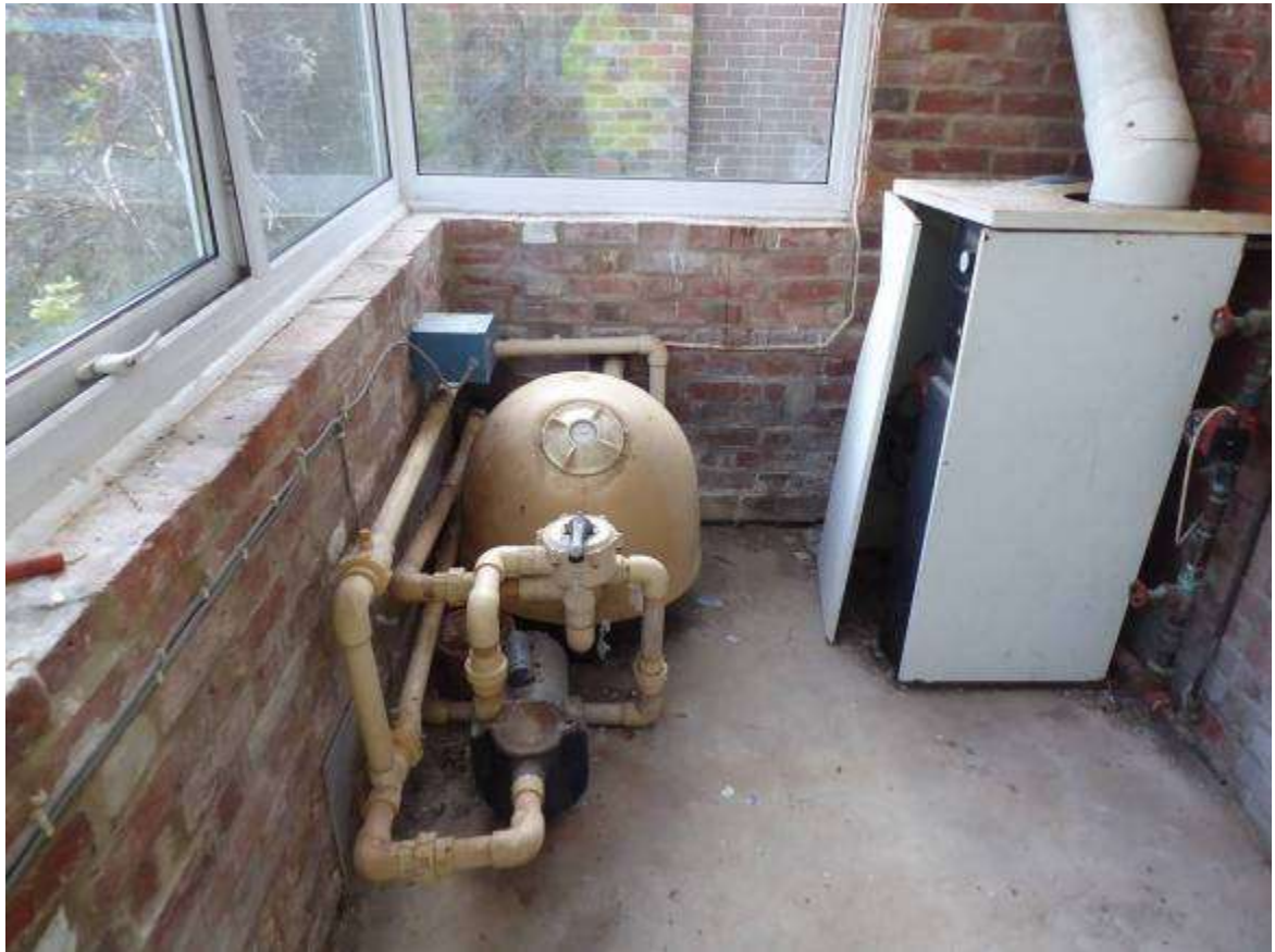
Fig 4.9: Swimming pool plant room
