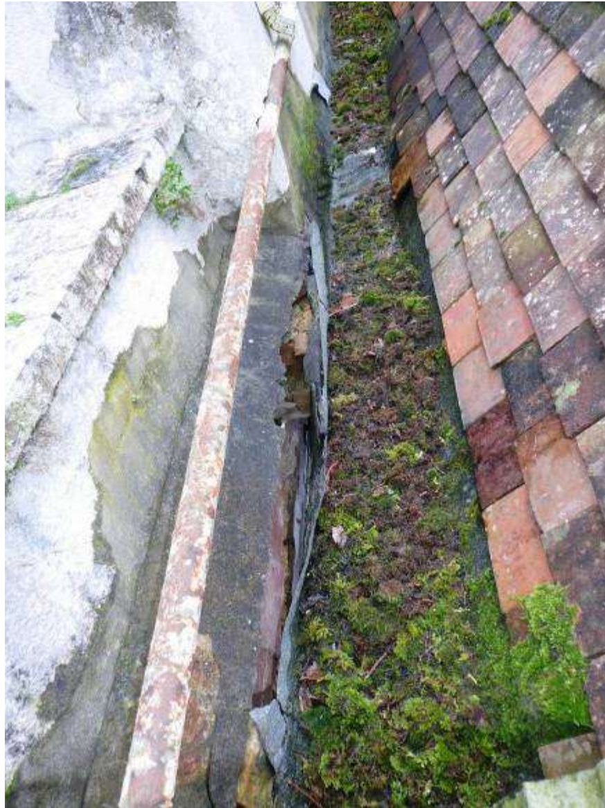
Fig 3.4.6: Failed valley gutter to north side of service block
