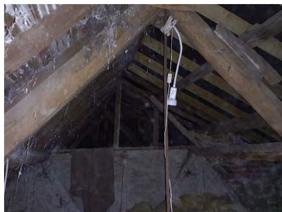
Figure 32: The remaining 3m of the loft was not safe to access
