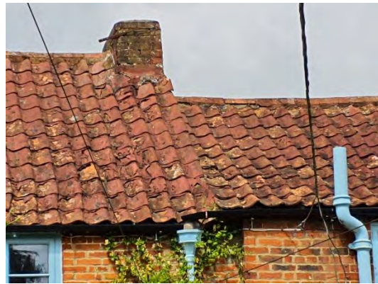
Figure 29: Potential gaps in the ridge tile mortar
