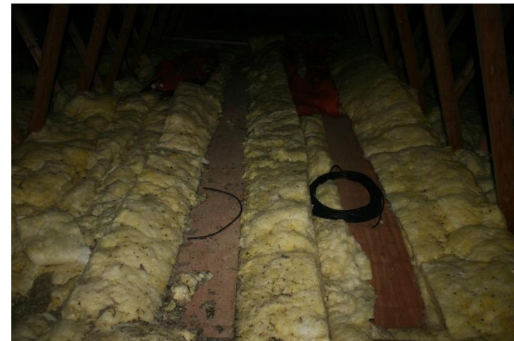
Photo 3: Bat droppings scattered in the loft.
