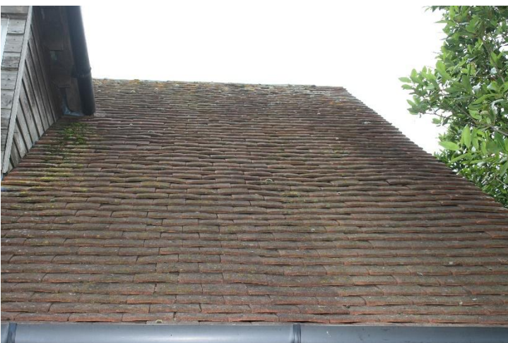
Photo 10: Lifted tiles on the annexe (B1).
