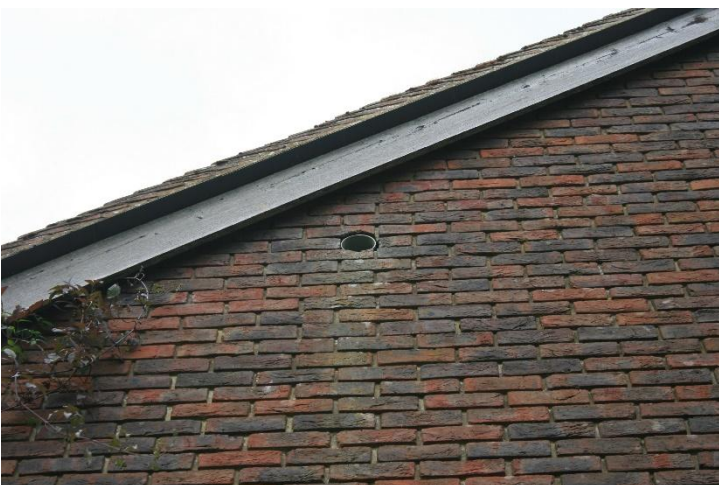
Photo 7: Gaps under the fascia on the west gable (B1).
