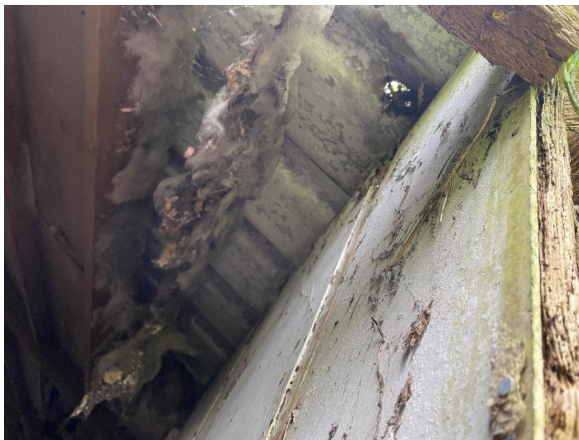
Photograph 8: Hole in the roofing sheet of B1
