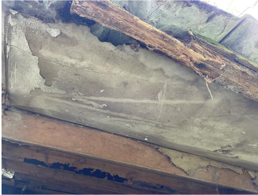
Photograph 9: Gap between roofing sheet and boarding in B1
