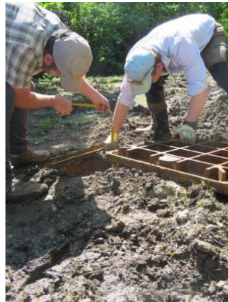
Private Manhole Chamber for Surface Water
