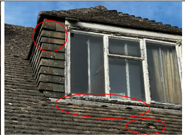
Figure 9: Lifted lead flashing, roof tiles and hanging tiles
