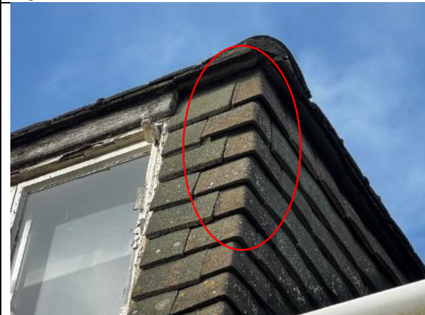
Figure 4: Lifted hanging tiles on eastern dormers on B1
