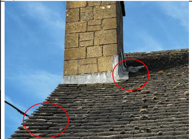
Figure 6: Lifted roof tiles and lead flashing on east elevation
