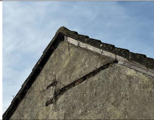
Figure 20: Superficial cracks on east gable of B3
