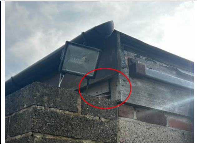
Figure 15: Gap in fascia on north-east corner of B2
