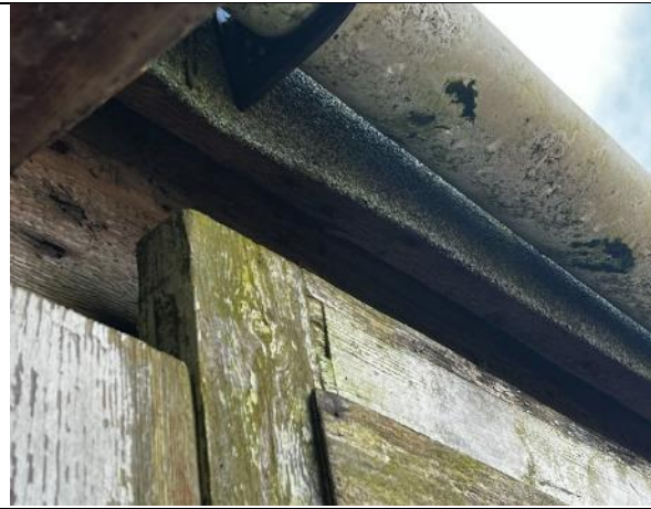
Figure 14: Lifted felt and fascia on B2
