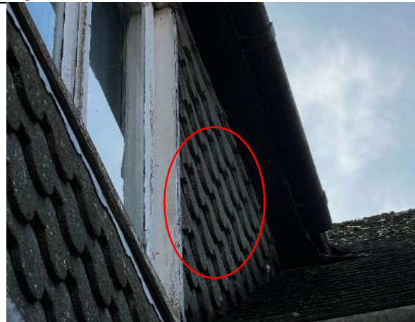
Figure 5: Lifted hanging tiles on west elevation of B1
