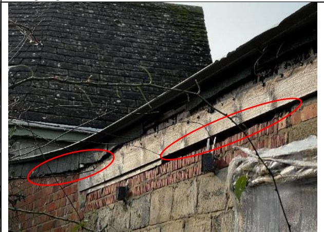
Figure 12: Lifted fascia and felt on east elevation of B2
