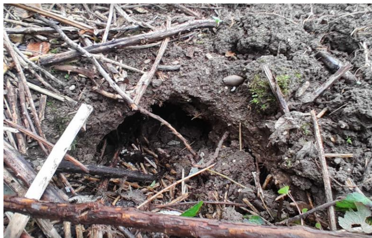
Figure 10 - View of partially collapsed hole located down the east of the site where the hedgerow was removed.
