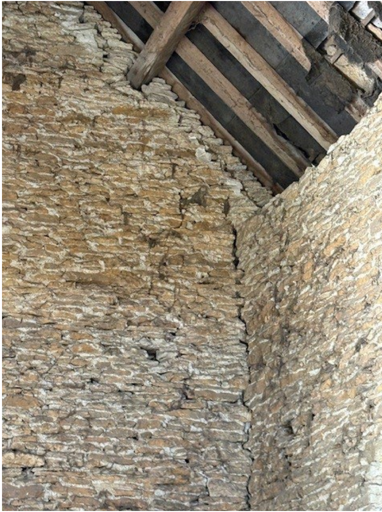
PLATE 13 -- CRACK IN CORNER
