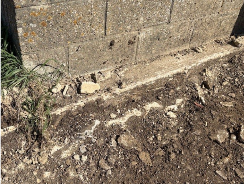
PLATE 21 -- WALL AND FOUNDATION
