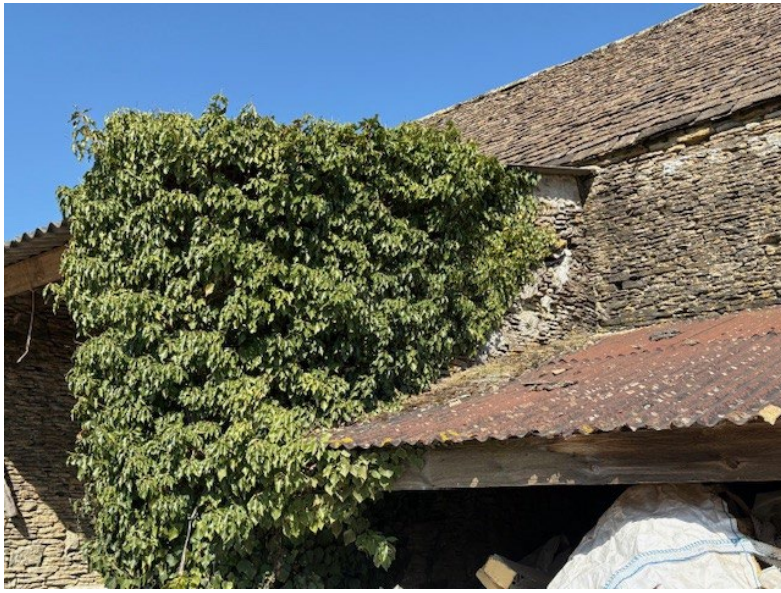
PLATE 19 -- PARTLY COLLAPSED WING WALL
