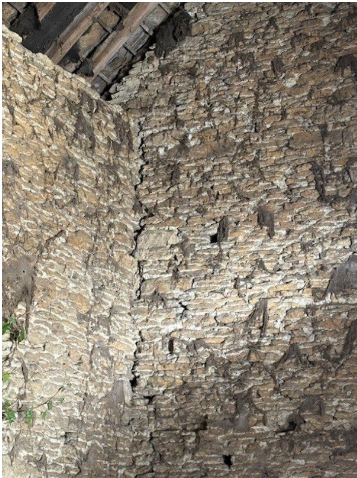
PLATE 12 -- CRACK IN CORNER
