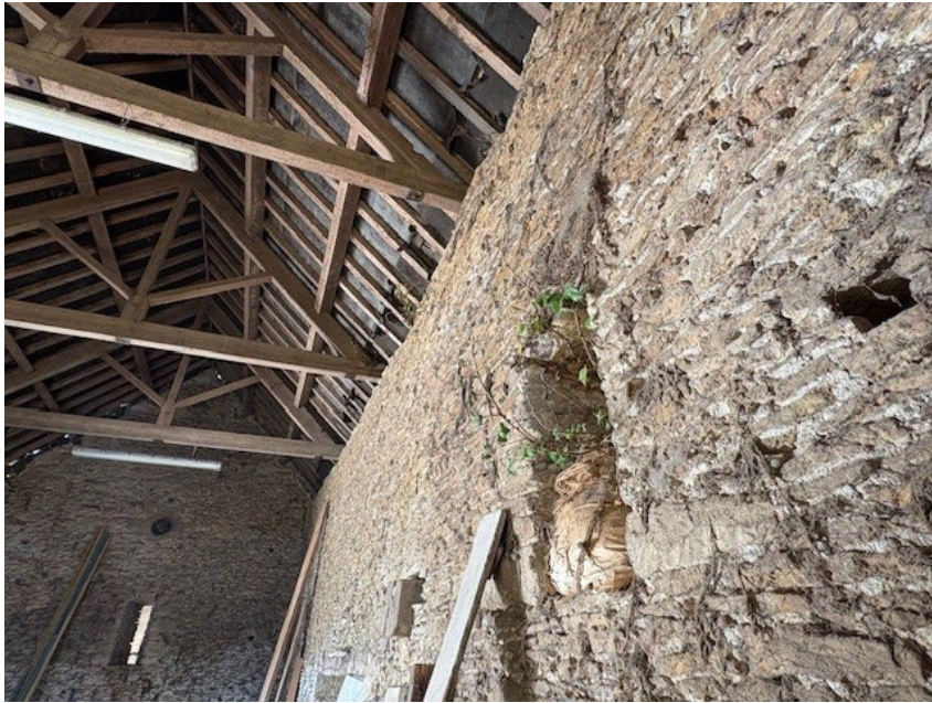
PLATE 11 -- OUTWARDS LEAN OF NORTHERN WALL
