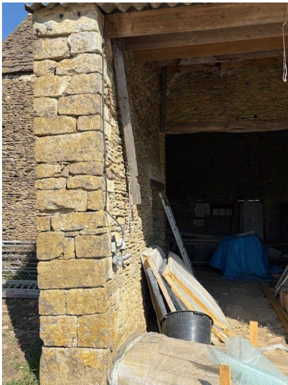
PLATE 18 -- BADLY LEANING WING WALL
