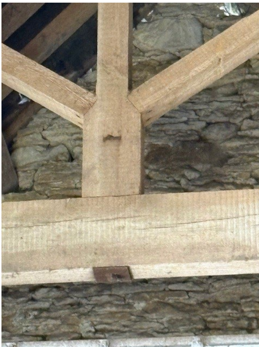
PLATE 08 -- TIGHT TRUSS JOINT AND BOTTOM TIE
