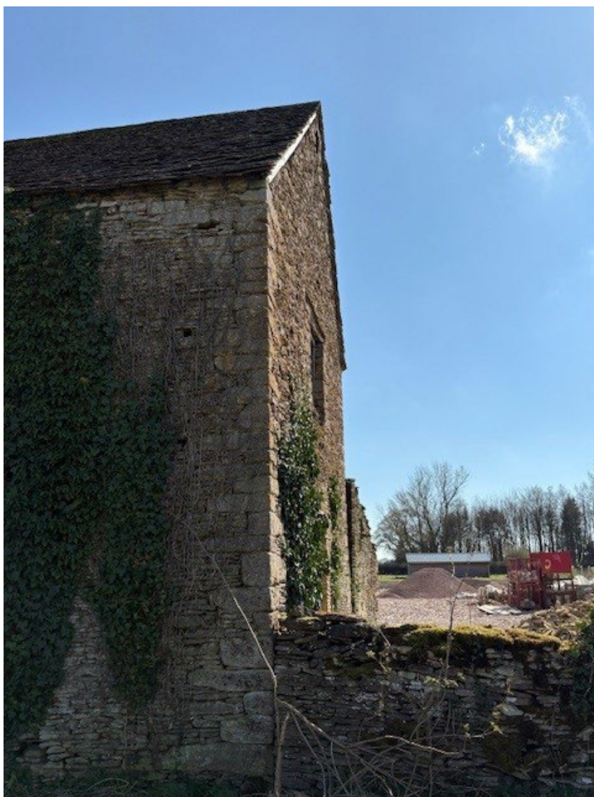
PLATE 10 -- OUTWARDS LEAN IN TOP OF EASTERN WALL
