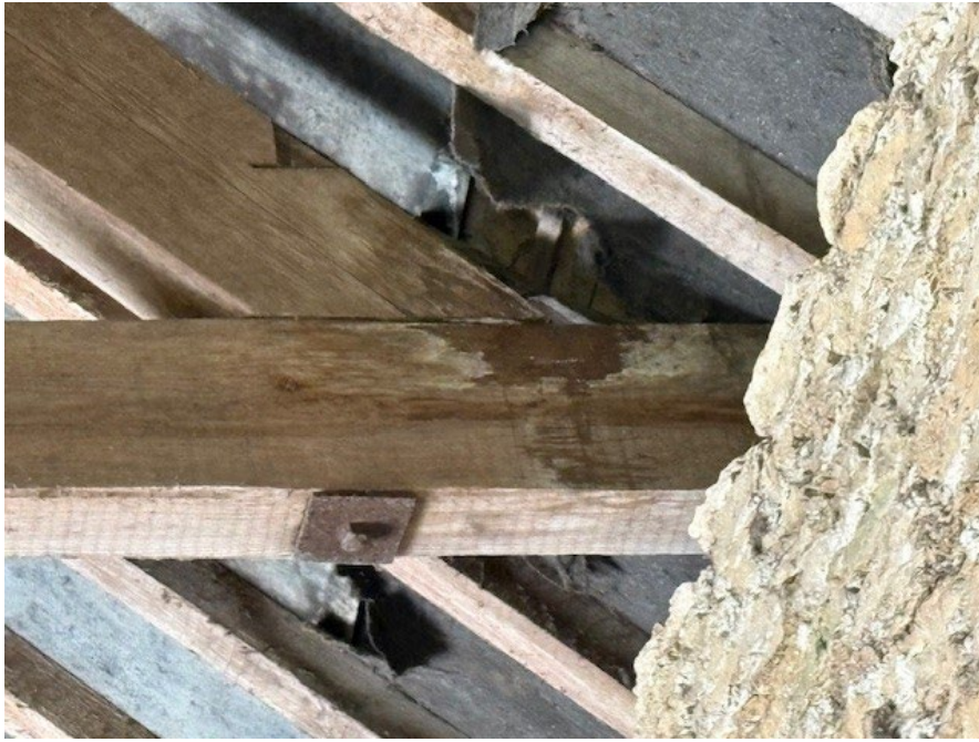
PLATE 06 -- NOMINAL DAMP PENETRATION
