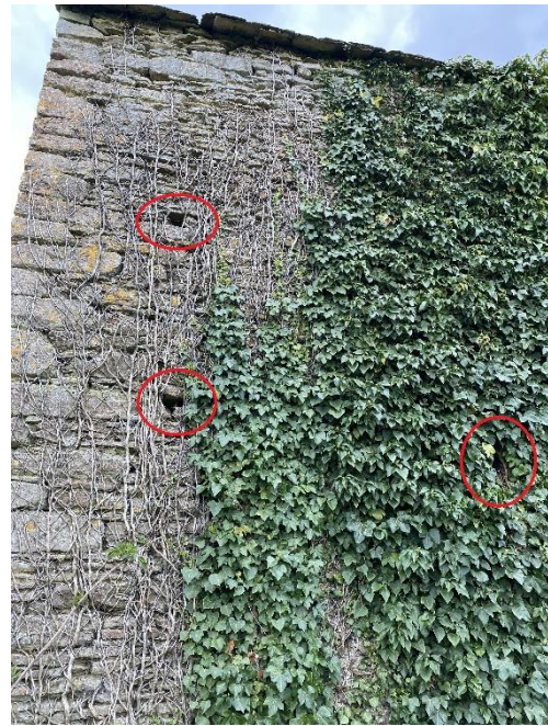
Photograph 4: Dense Ivy and PRFs on northern wall.
