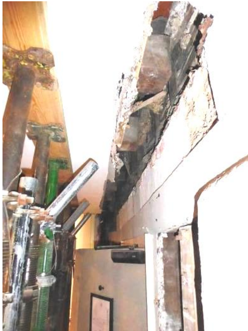
Fig 3.2.2: Position of failed bear plate
