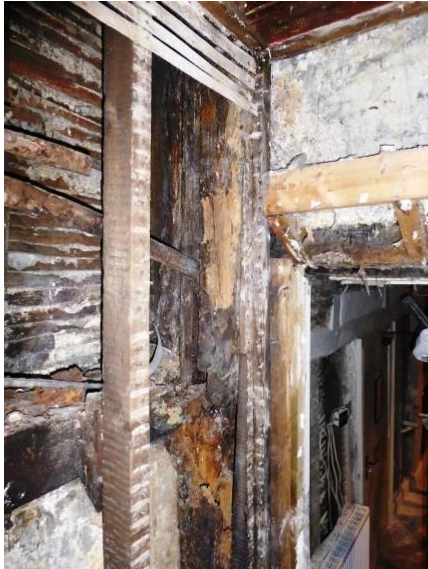
Fig 3.2.3: Decayed main timber post
