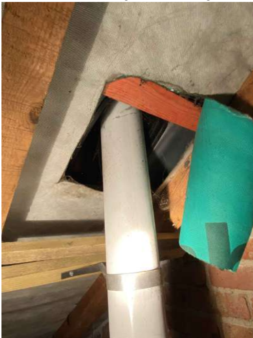
Plate 15: Gas flue exiting the roof through removed tile.
