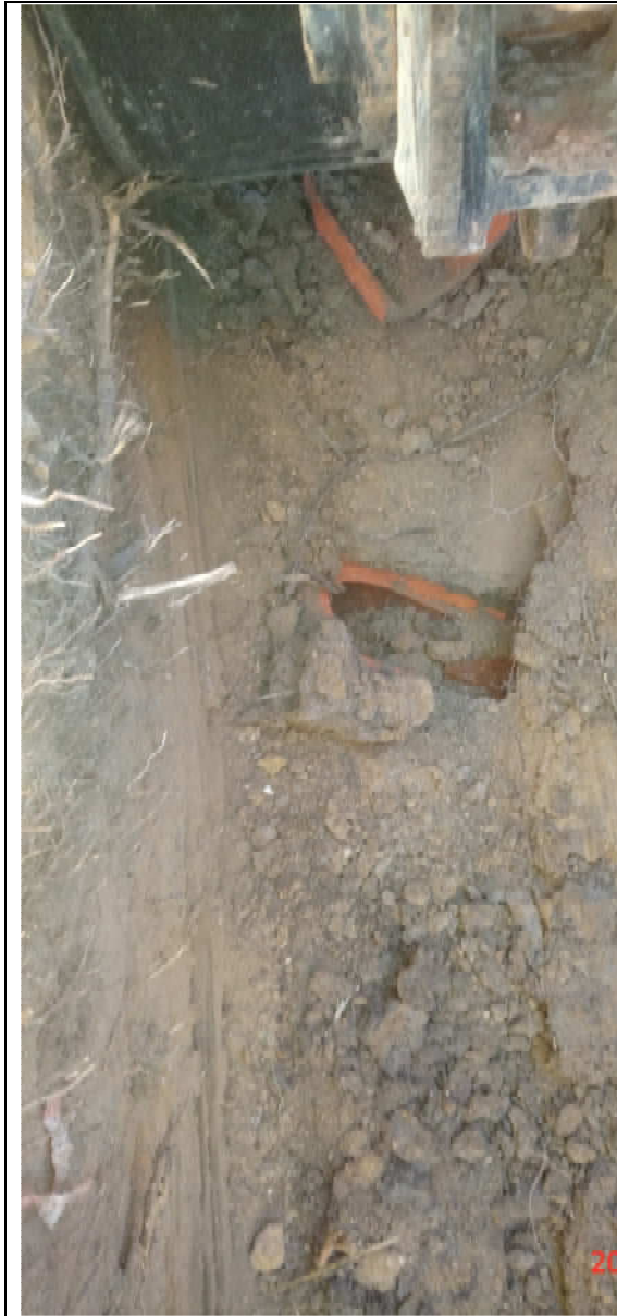
L/R Wagtails, Alderbury – Existing Land Drains
